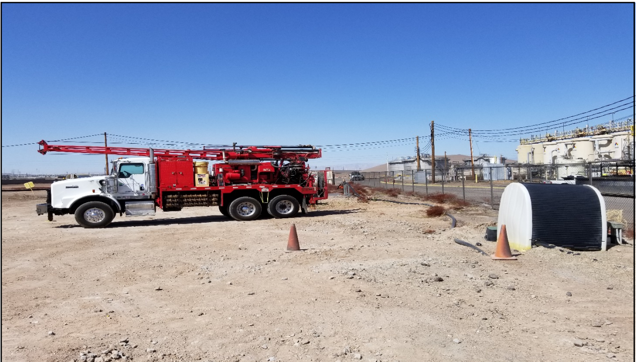
Facing West: Former UFIW-01, UFIW-02, UFIW-03 and UFIW-04 locations after well abandonment.
