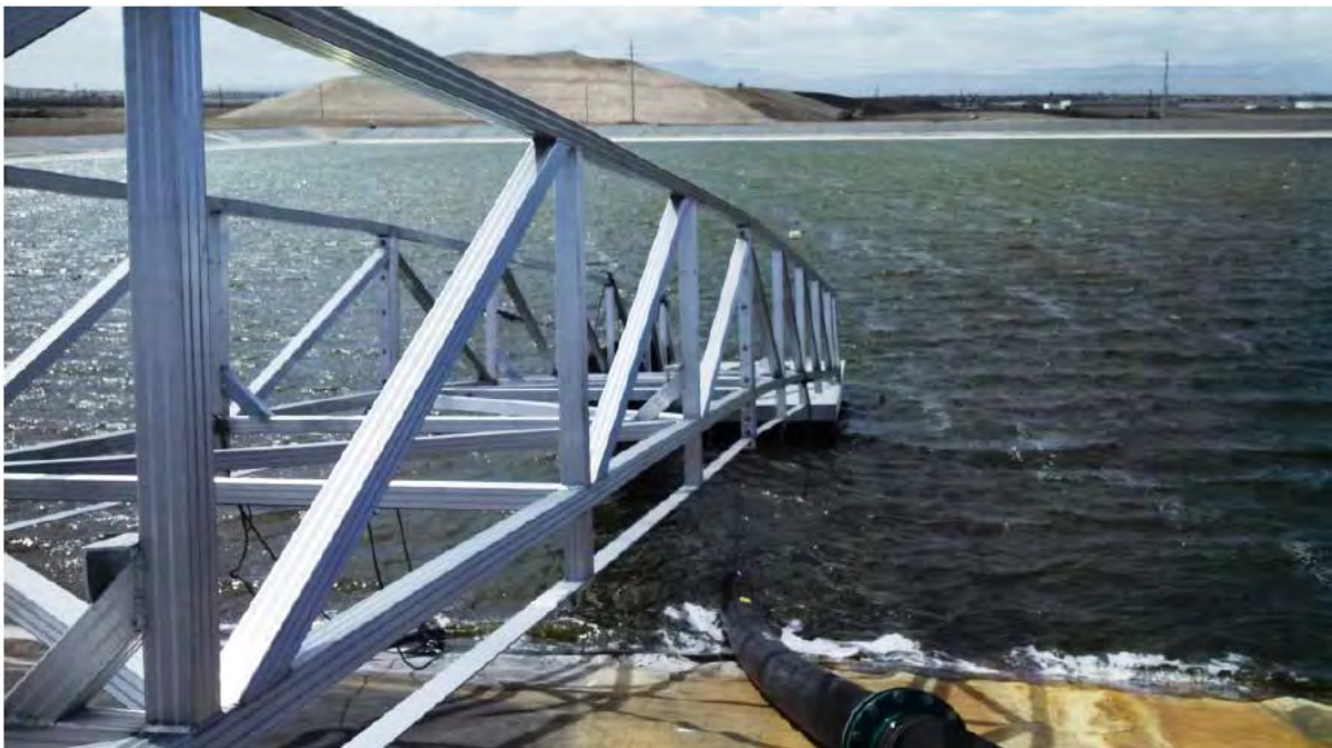
Photo 6: Facing west. View of the completed floating dock control arm and HDPE intake pipe.
