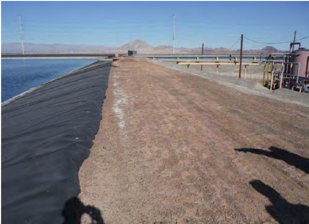
Photo 1: Facing north. View of eastern berm roadway prior to construction and excavation activities.
