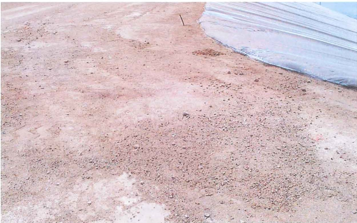
Fig. 2. Post clean-up picture (8/2/13) of the top of the MN2 Pond berm where the spill was generated.
