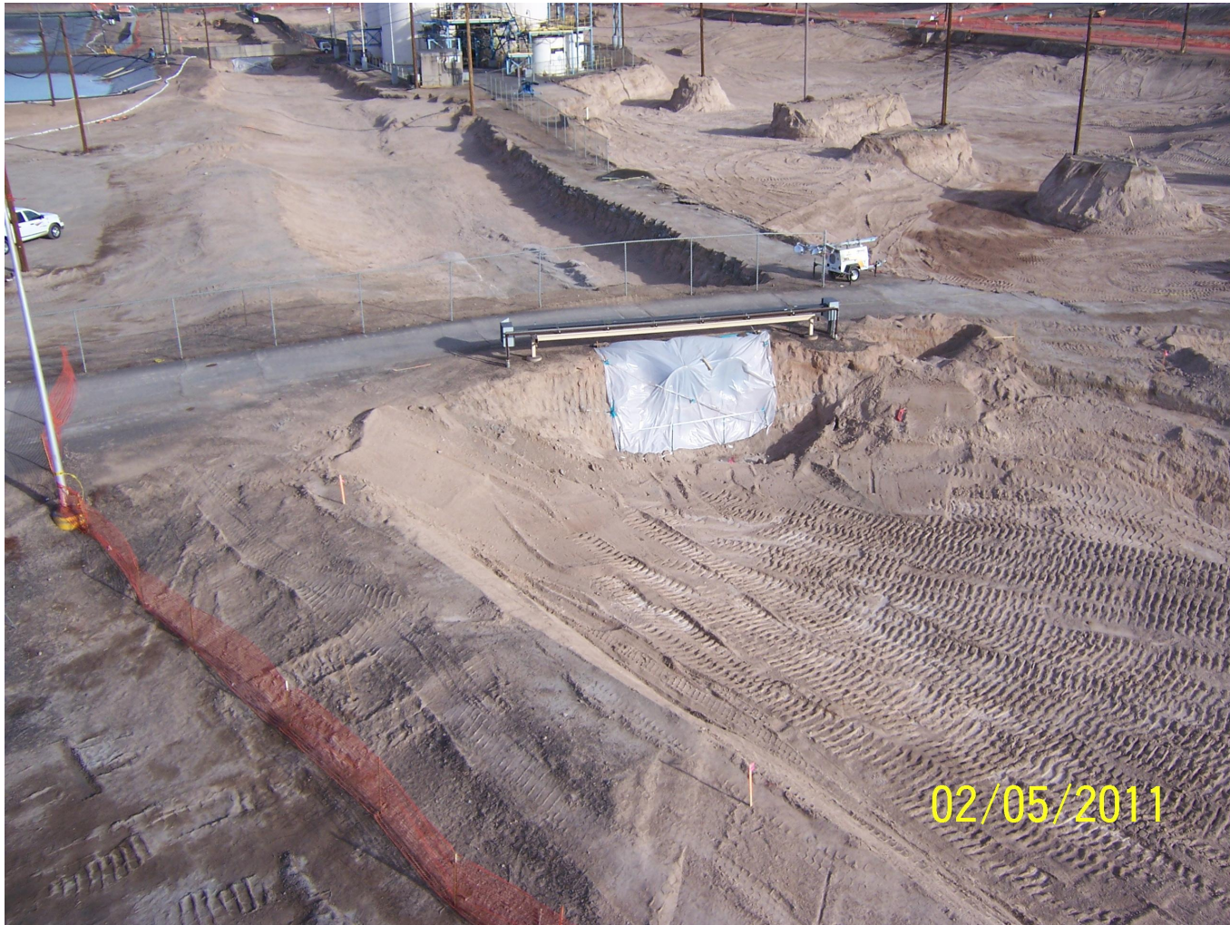
RZ-E- 6 ACM Excavation with Orange Fence Drainage Pipes had to Remain in place Until Utilities were Moved
