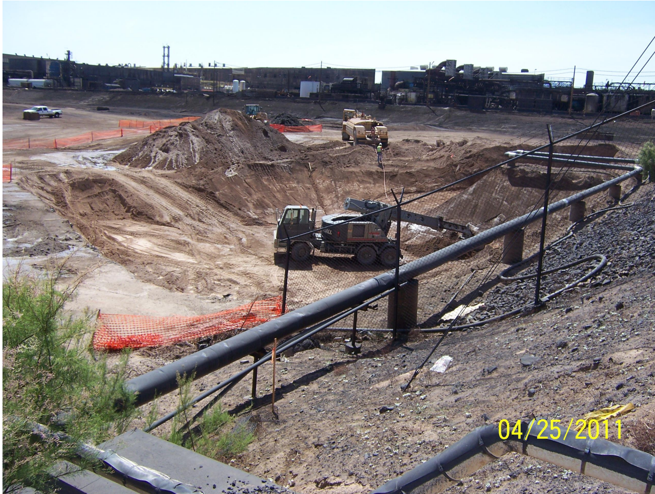
South RZ-C- 44 Polygon Excavation A Gradeall was utilized to protect the in place Utilities
