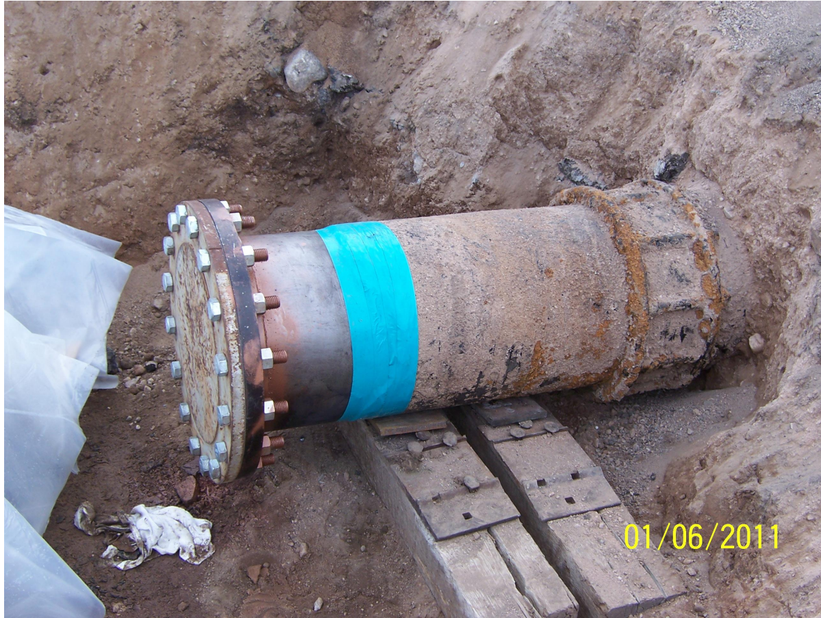
South RZ-C- 45B Emergency Repair of 20" Water Line This water line was deteriorated to the point it started leaking with out being hit
