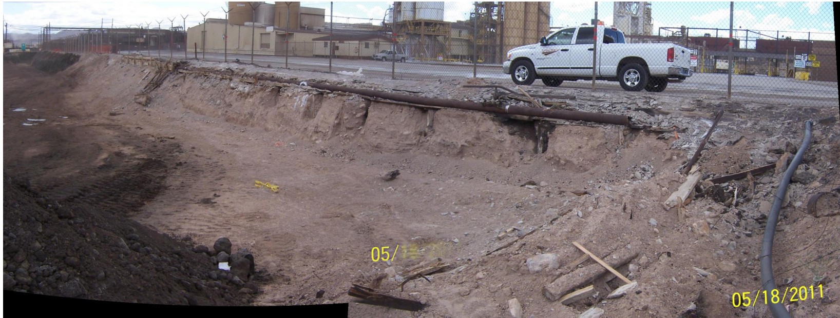
South RZ-C- 24 & 26 To be removed Pipes with Oil and Box Structure
