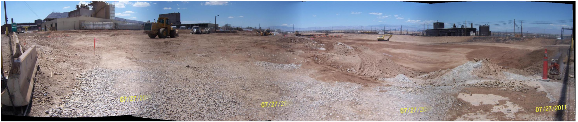
South RZ-C- 27 Backfilled to Grade Next Step is to finish Grade the Area
