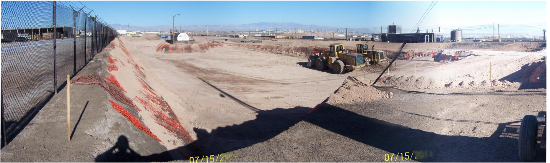
South RZ-C- 27 Partial Backfill Note Orange Fence Placed on Slopes to denote Boundary of Polygon Excavation
