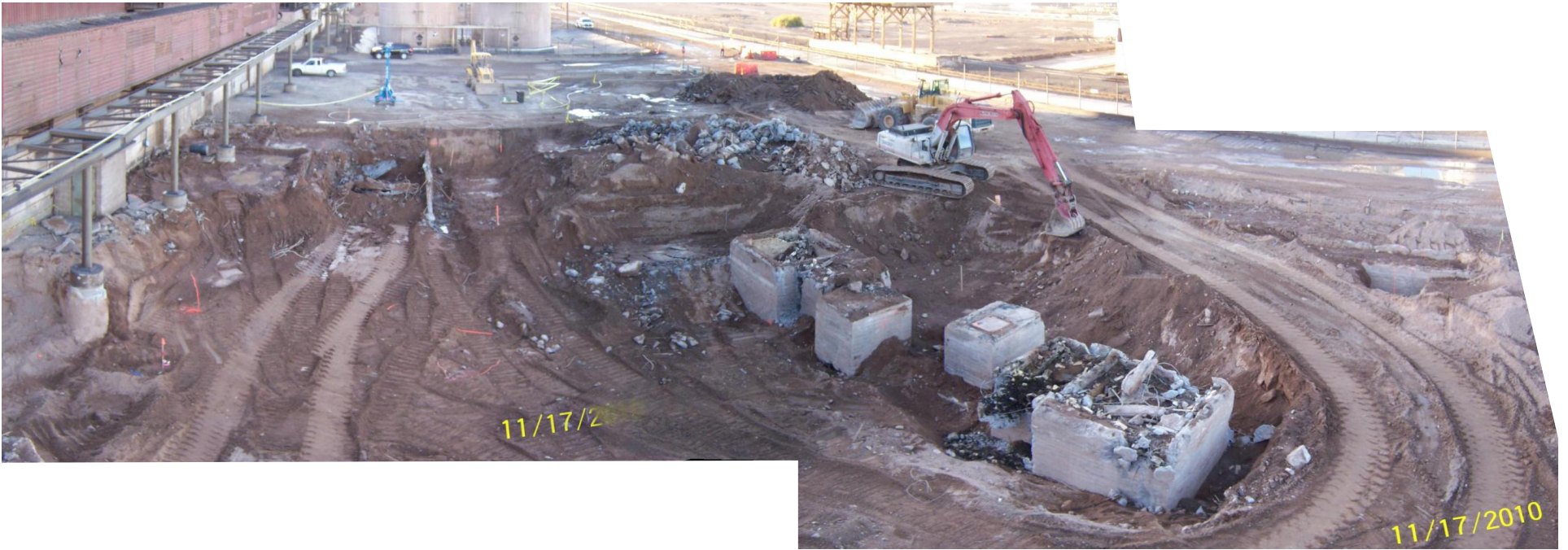
North Side of Unit Building #3 Found Hidden Foundations
