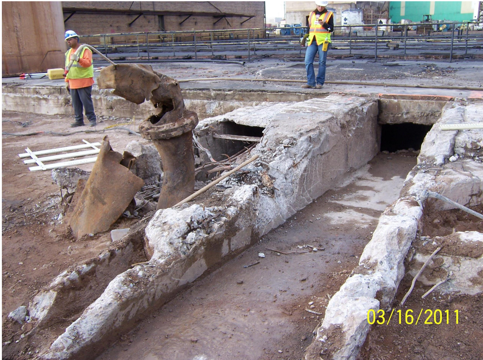
RZ-B-19,20,21 Concrete Tunnels that were Cleaned Out Sealed Off and left in place
