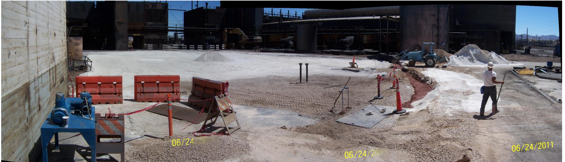
RZ-B-19,20,21 Area Backfilled with Chat and Piping Installed by Tronox for New Addition
