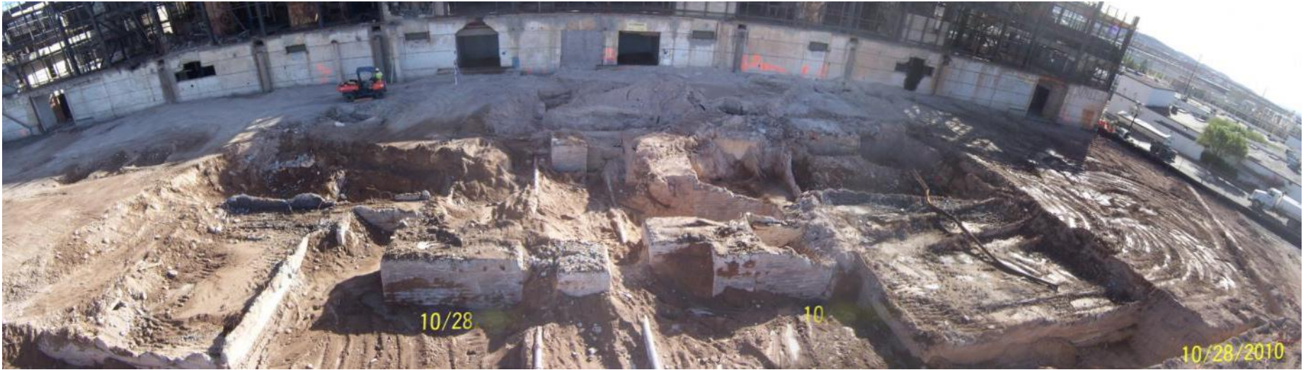
North Side of Unit Building #1 Found Hidden Foundations
