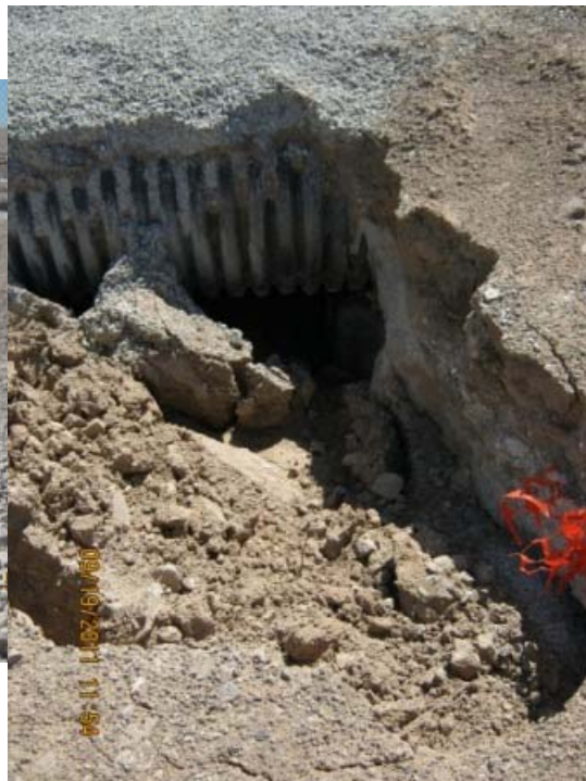
Area 2: Northwest corner – Culverts were temporary when road was installed. They are to be removed and flow from offsite diverted back to western property to minimize any onsite erosion. We are working with Landwell/BMI to have them removed.
