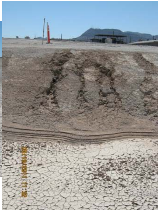
Area 7: RZ-D-17B. Will install directional berm(s) to flow into channel at designated location. Slope at inflow will include placement of nonwoven geotextile with 12" of 6" angular stone.
