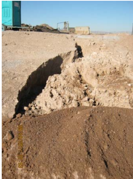
Area 6: West Side of New Drainage Channel. Will install directional berm(s) to flow into channel at designated location. Slope at inflow will include placement of nonwoven geotextile with 12" of 6" angular stone.
