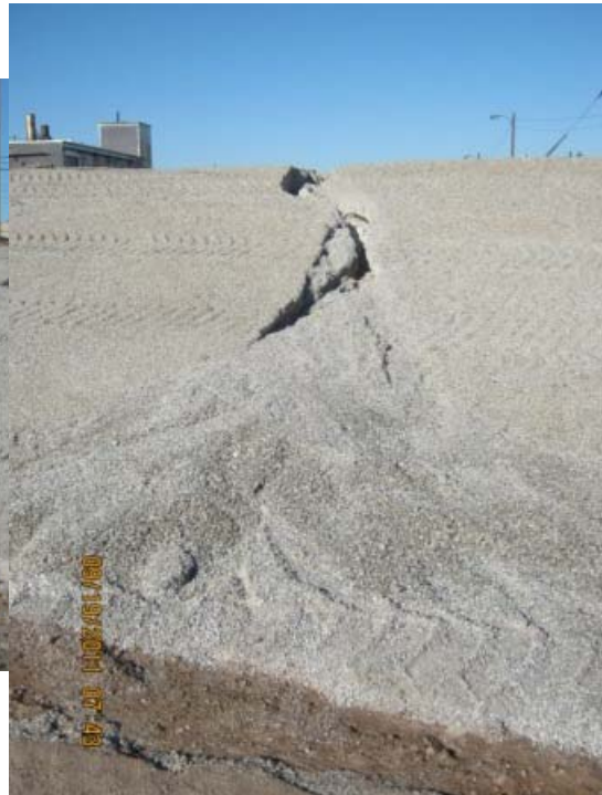
Area 5: RZ-E-14A. Runoff from roadway- Will install directional berm(s) to flow into channel at designated location. Slope at inflow will include placement of nonwoven geotextile with 12" of 6" angular stone.
