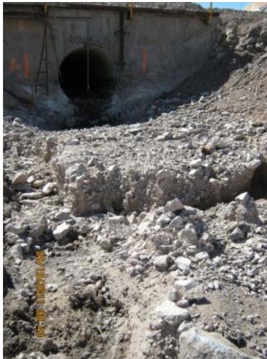
Area 9: Outfall 1. Design calls for 4 ft thick 24" Riprap which is in the process of being installed.
