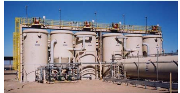
Biological Treatment Plant for Groundwater
