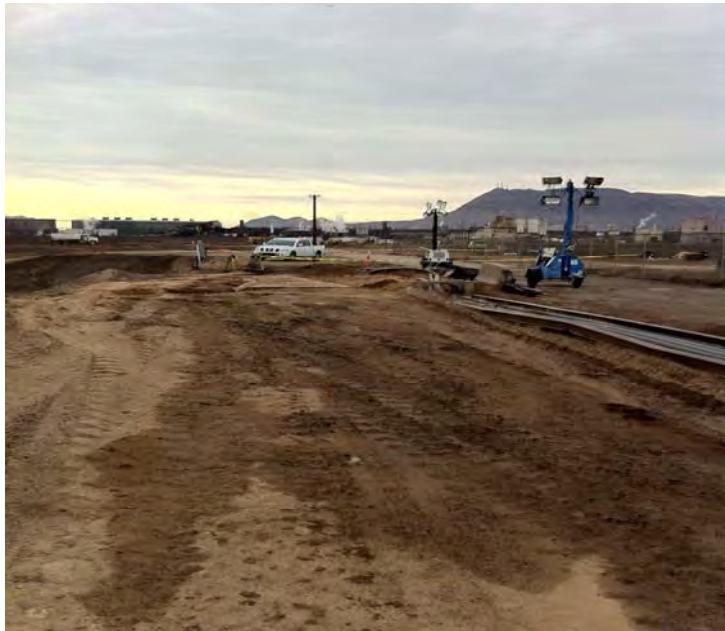
Photograph 2 View from just north of the damaged process lines looking towards the south.
