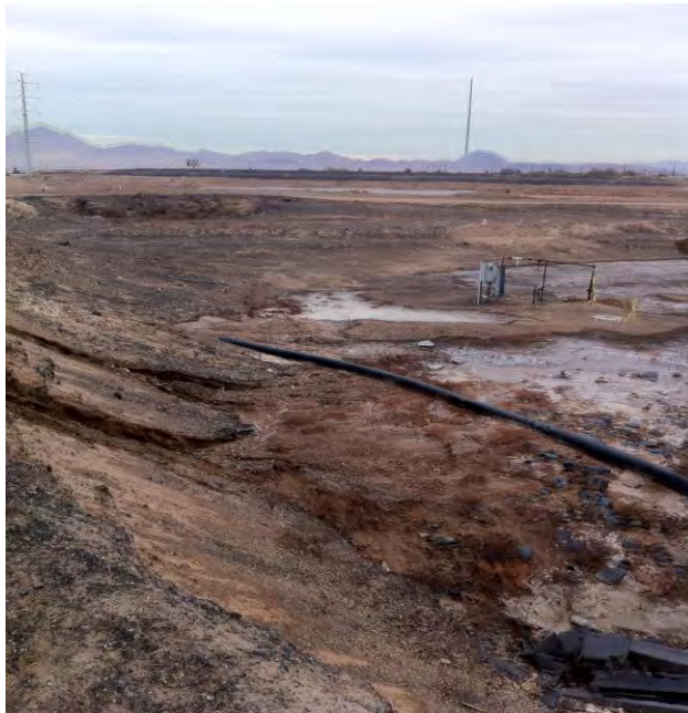
Photograph 4 View looking north just east of the damaged process lines. Soil sample S-1 was collected approximately 5 feet west of the grey well control box shown in the photo.
