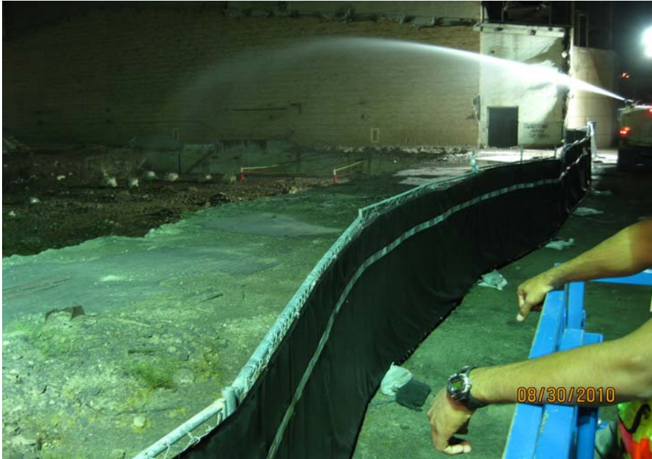
LVP water truck helping wet the work area. Looking south from observation lift.
