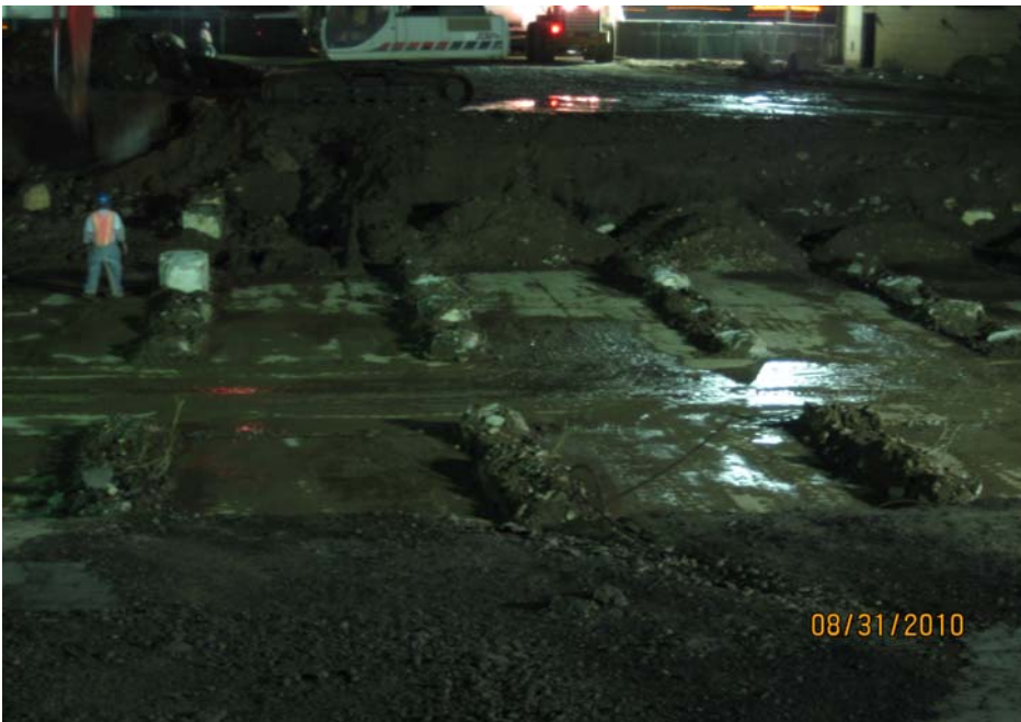
Floor at end of day. There will be shovel work to finish the floor.
