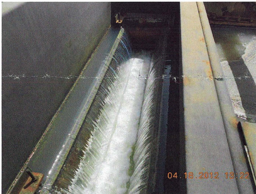
Fig. 9 – DAF Effluent (to filter)
