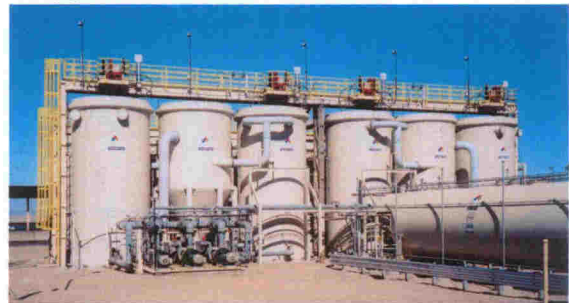
Biological Treatment Plant for Groundwater
