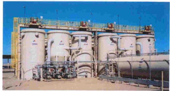
Biological Treatment Plant for Groundwater
