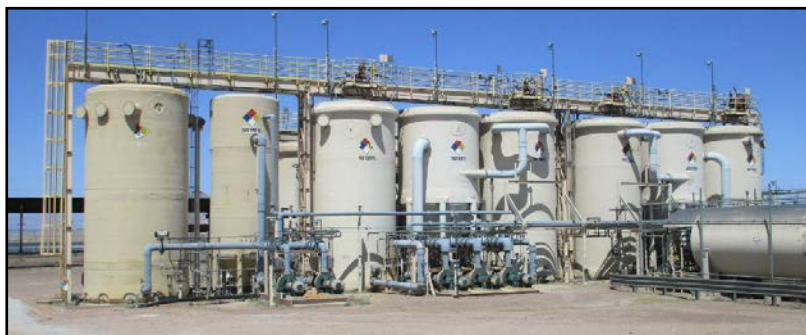
Groundwater Treatment System at the NERT Site
