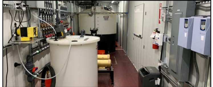
Injection and Extraction System Equipment for a NERT Treatability Study
