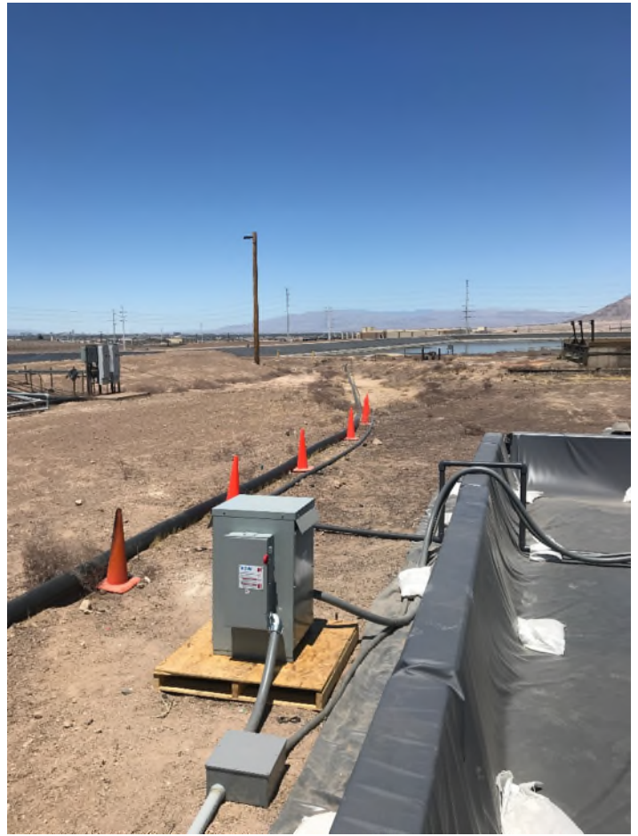
New transformer for electrical connection.
