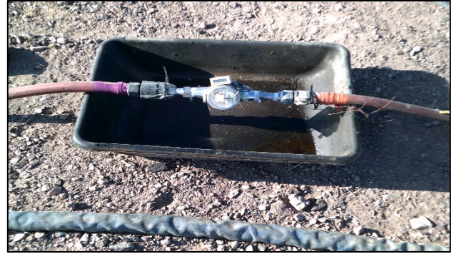
10. Flowmeter used for groundwater extraction.
