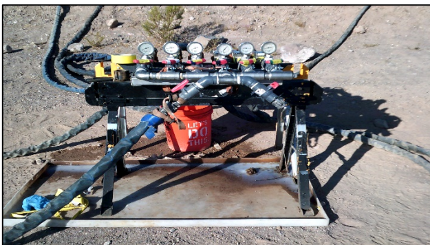
15. Injection manifold (inlet).
