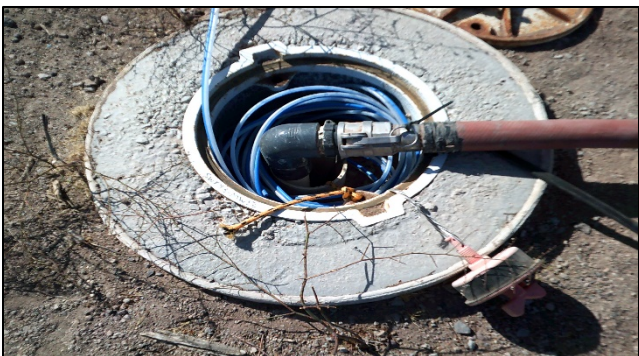
8. Extraction well. 1.5" PVC attached to a 4" extraction pump below grade.
