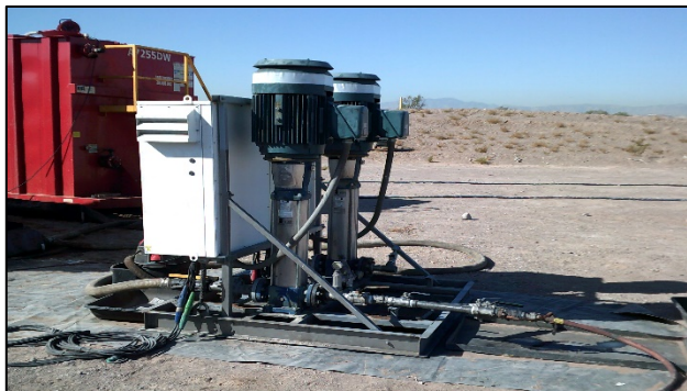
13. Dual skid mounted centrifugal injection pumps.
