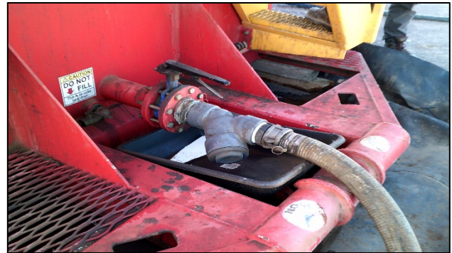
12. Three-inch Y-strainer to filter substrate prior to passing through injection system.
