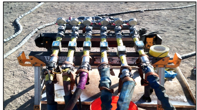
14. Injection Manifold (outlet).
