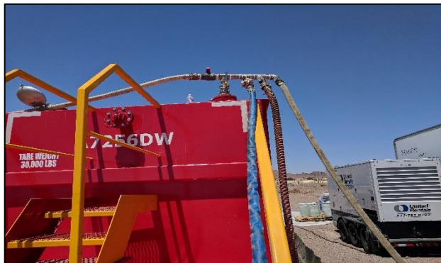
5. Extraction well manifold
