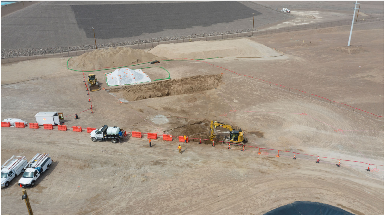
Photo 3: April 4, 2019. Excavation of the southwest and central portions of the non-ECA area. View to west.
