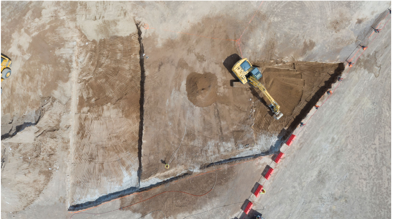
Photo 6: April 16, 2019. Excavation of the central portion of the non-ECA area. North at top of image.
