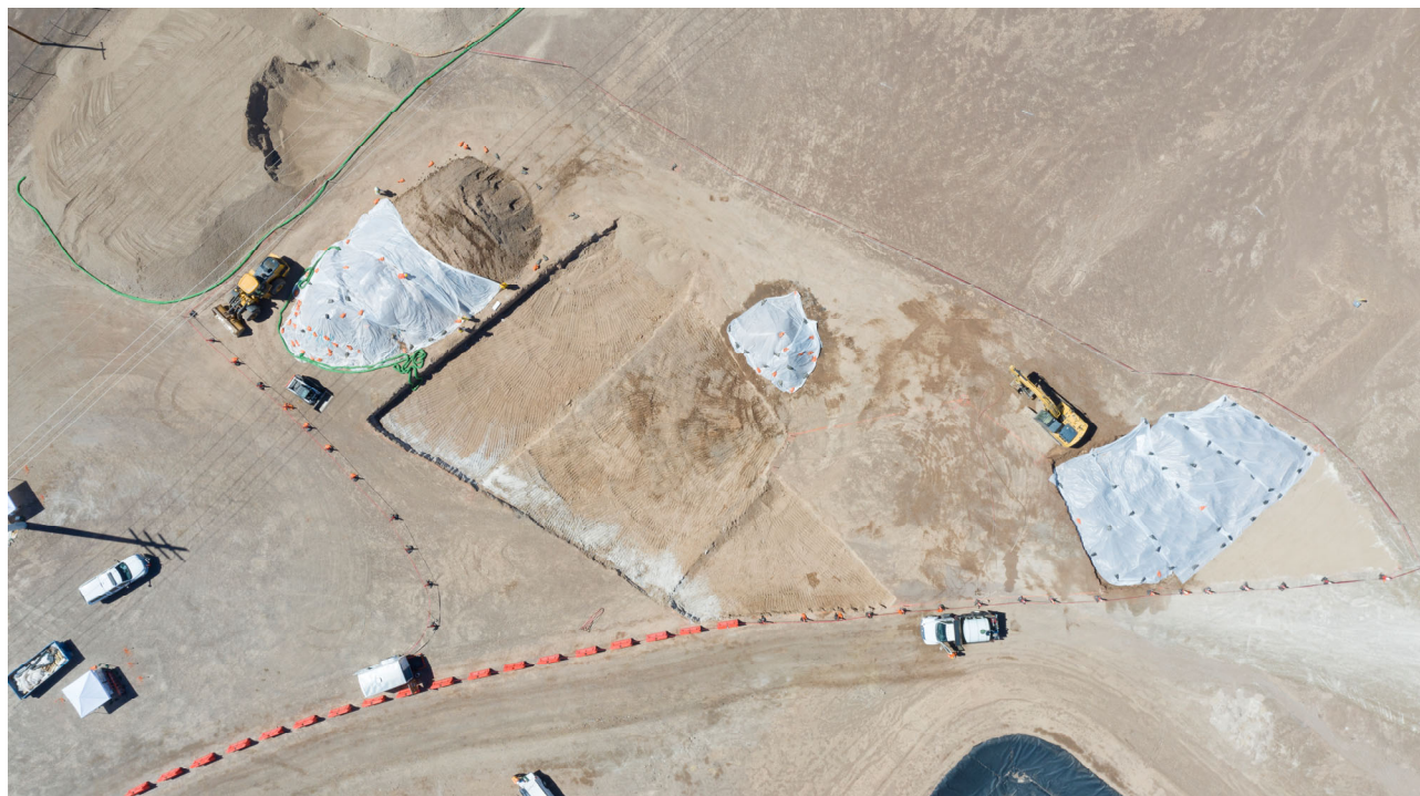
Photo 7: April 17, 2019. Excavation in central and northeastern portions of non-ECA area. The triangular ECA area (at right) has been backfilled and compacted.
