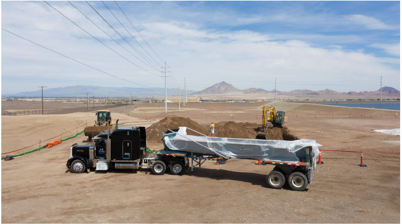
Photo 5: April 15, 2019. Excavation and removal of soil from the southwest portion of the non-ECA area. View to north.
