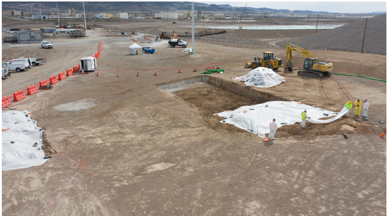
Photo 4: April 15, 2019. Excavation and removal of soil from the southwest portion of the non-ECA area. View to southwest.
