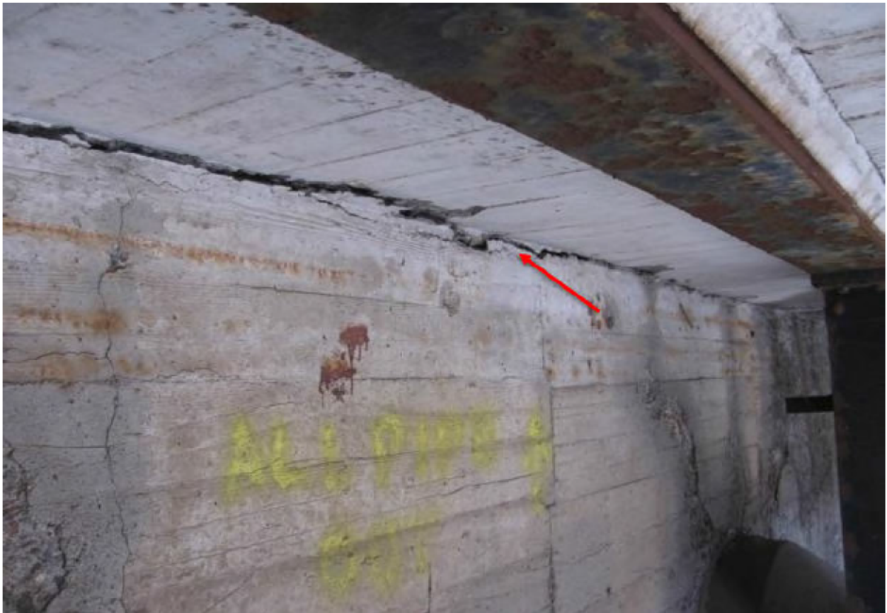
Figure 24: Cracking between the Unit 4 Cell Building north curtain slab and supporting partition wall
