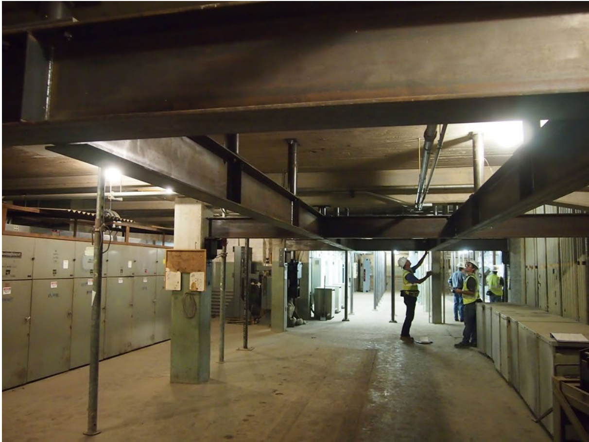
Figure 3: Structure in Basement of Substation Building
