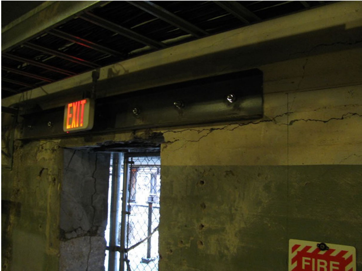
Figure 3: Medium Sized Cracks in Substation Building
