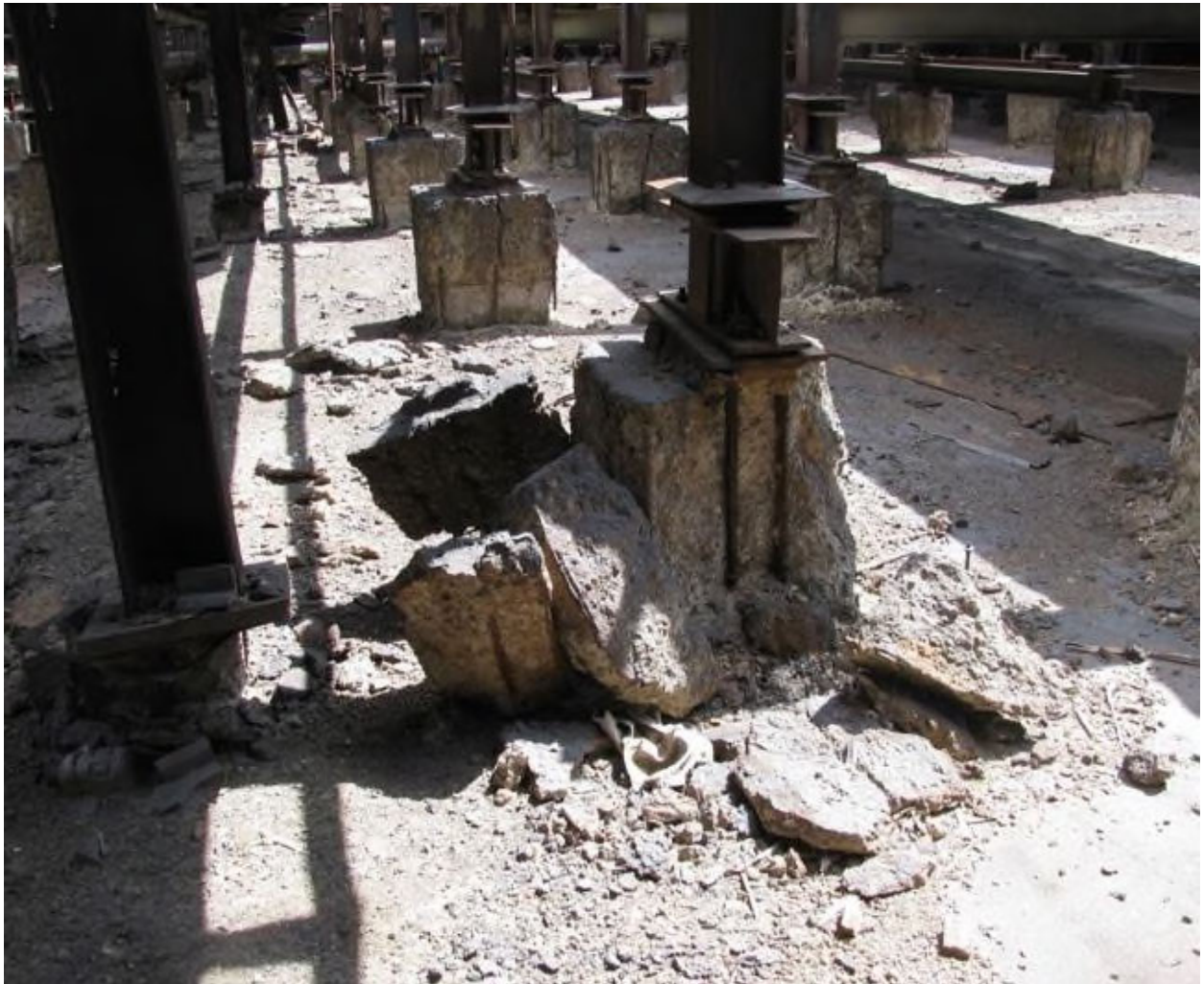
Figure 20: A crumbling Unit 4 Cell Floor column pedestal
