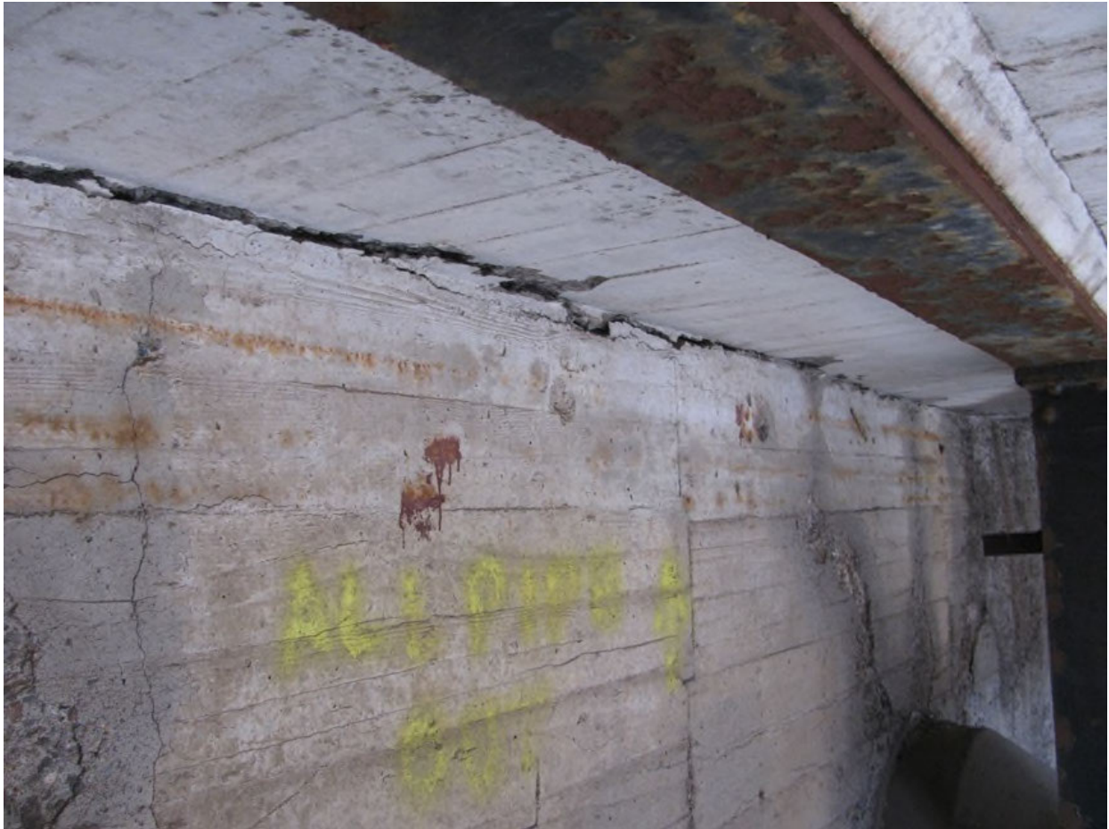
Figure 4: Large Sized Cracks in Substation Building
