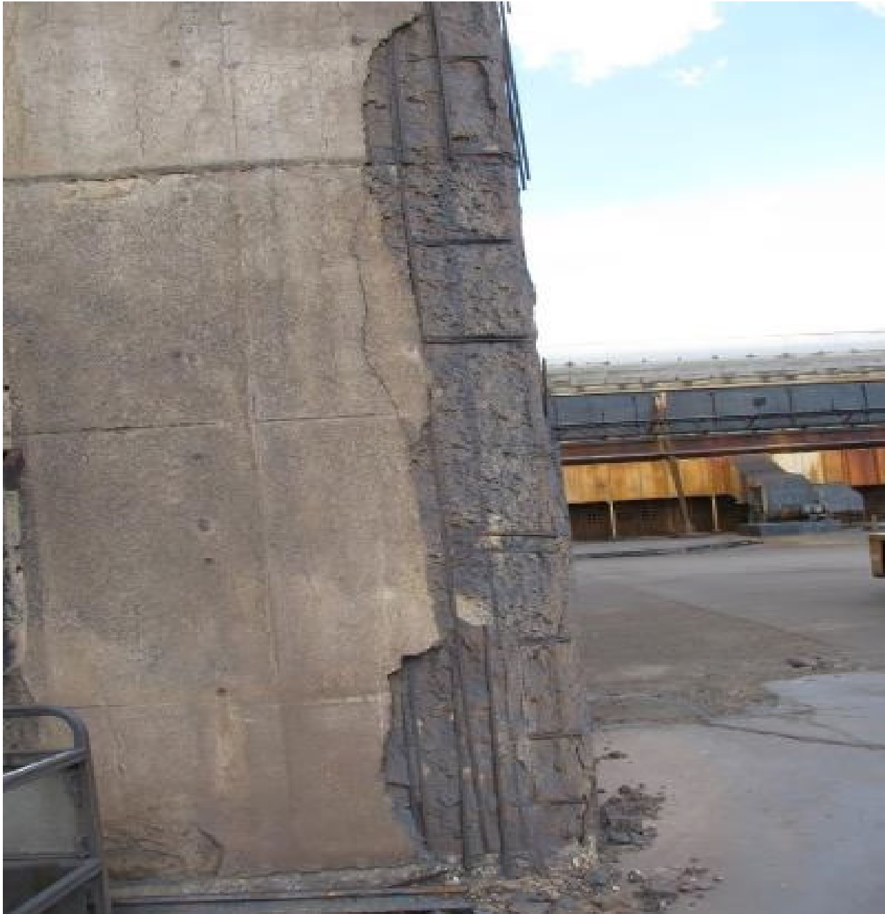
Figure 38: Unit 4 Wash Down Tower – spalling concrete near base
