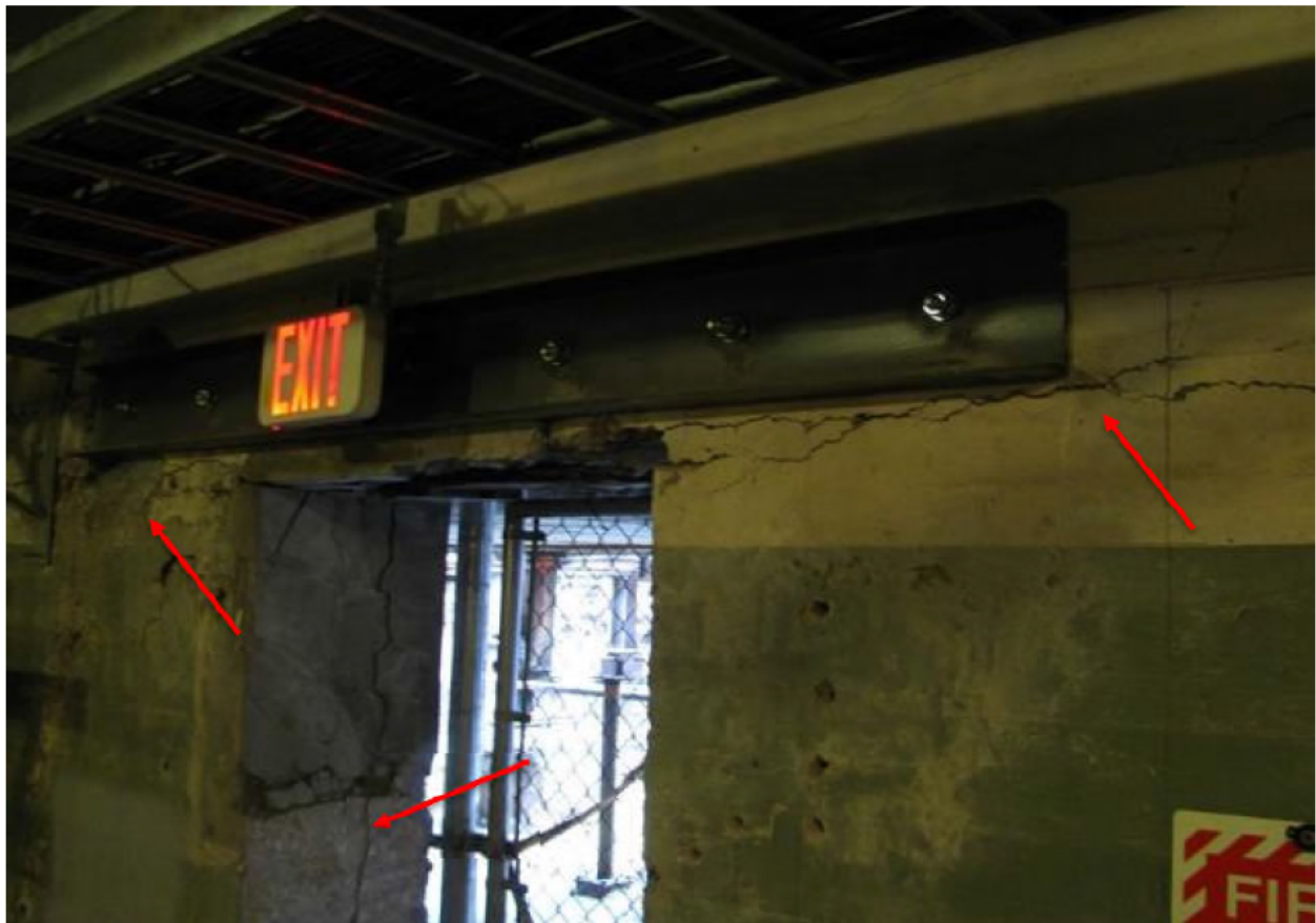
Figure 13: Horizontal cracks in Unit 4 Substation Building basement wall near eastern door, and vertical crack in the wall section at the door opening
