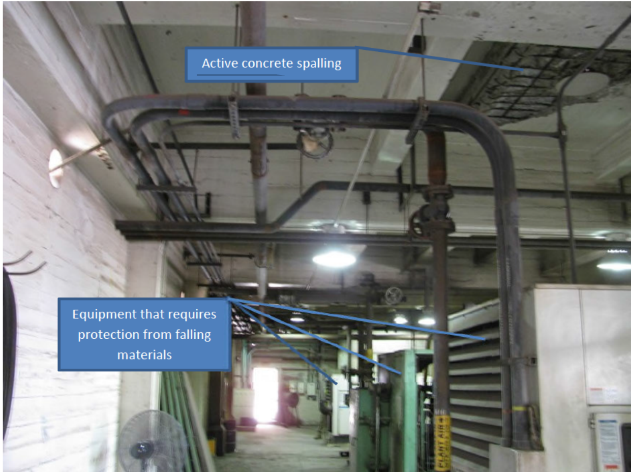
Figure 2: Some of the Tronox Equipment with Spalling Concrete Above
