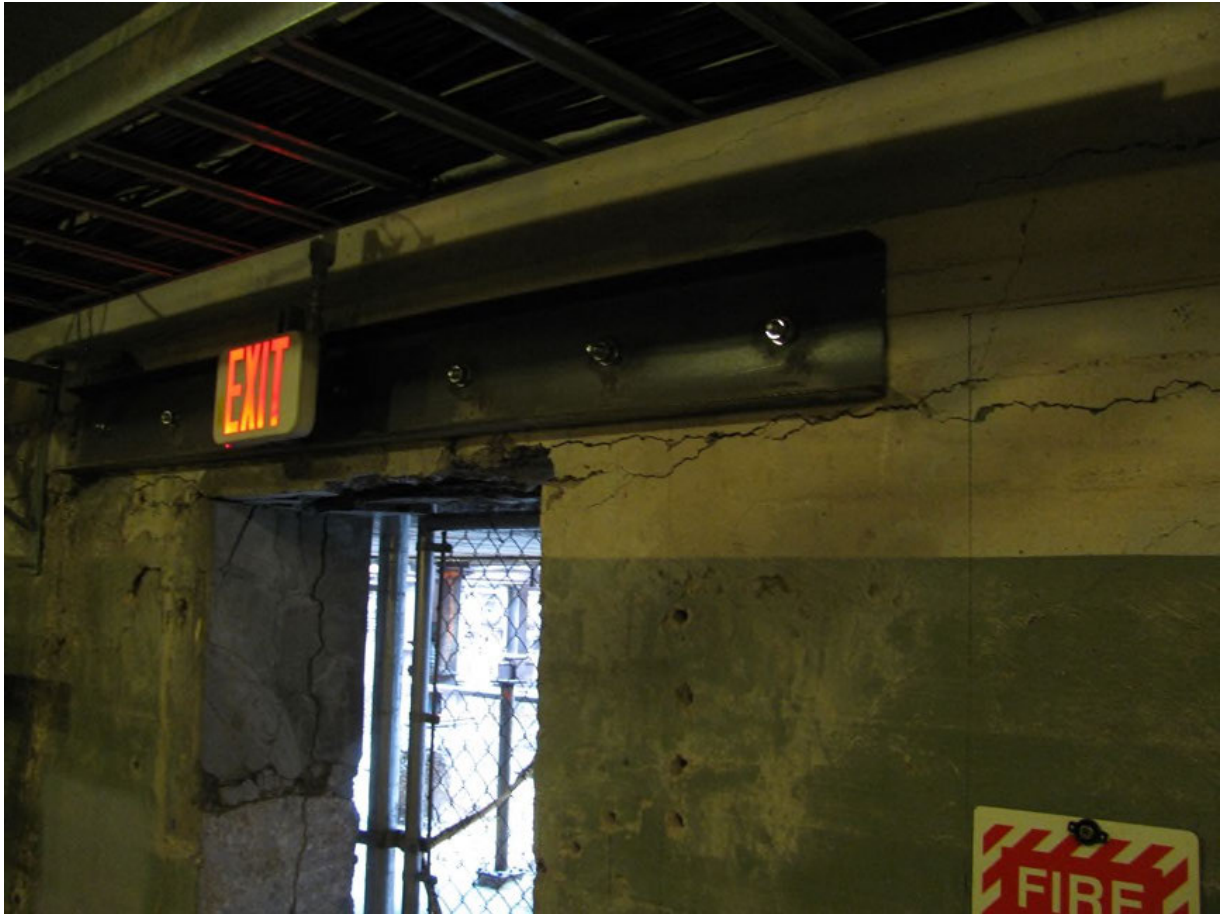
Figure 5: Existing Cracks in Basement of Substation Building at Eastern Doorway
