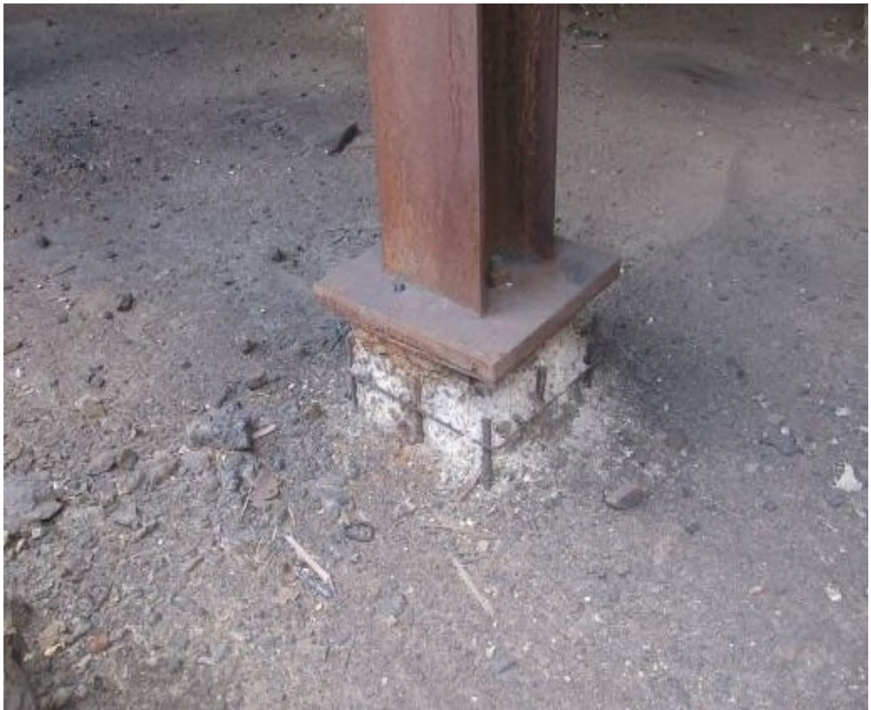
Figure 19: Unit 4 Cell Floor column pedestal, exposed rebar, severe spalling
