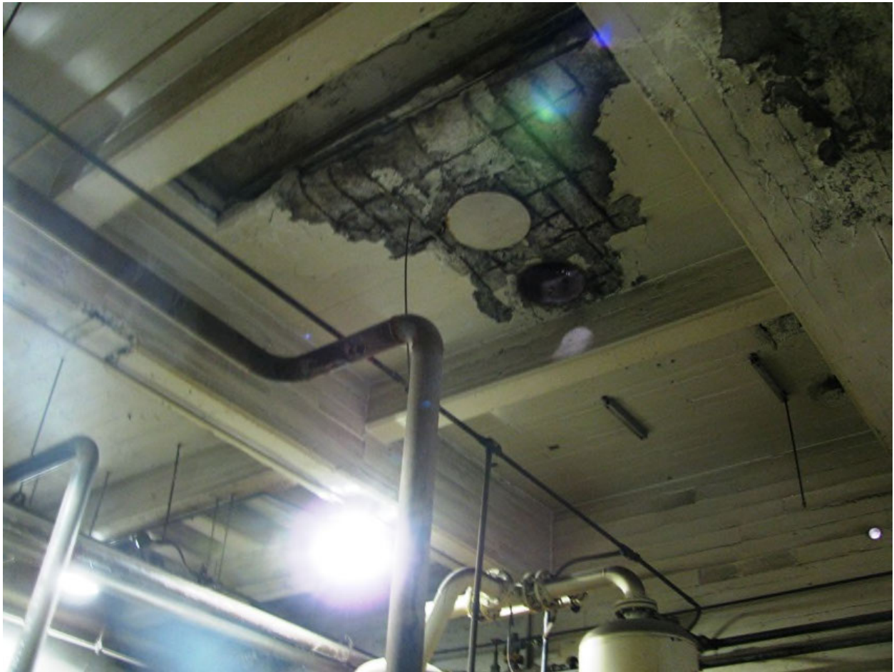
Figure 32: Spalling concrete above air dryer
