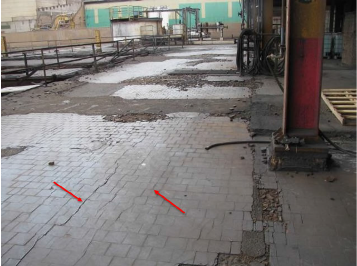
Figure 26: Unit 4 Cell Building curtain slab brick tile cracking
