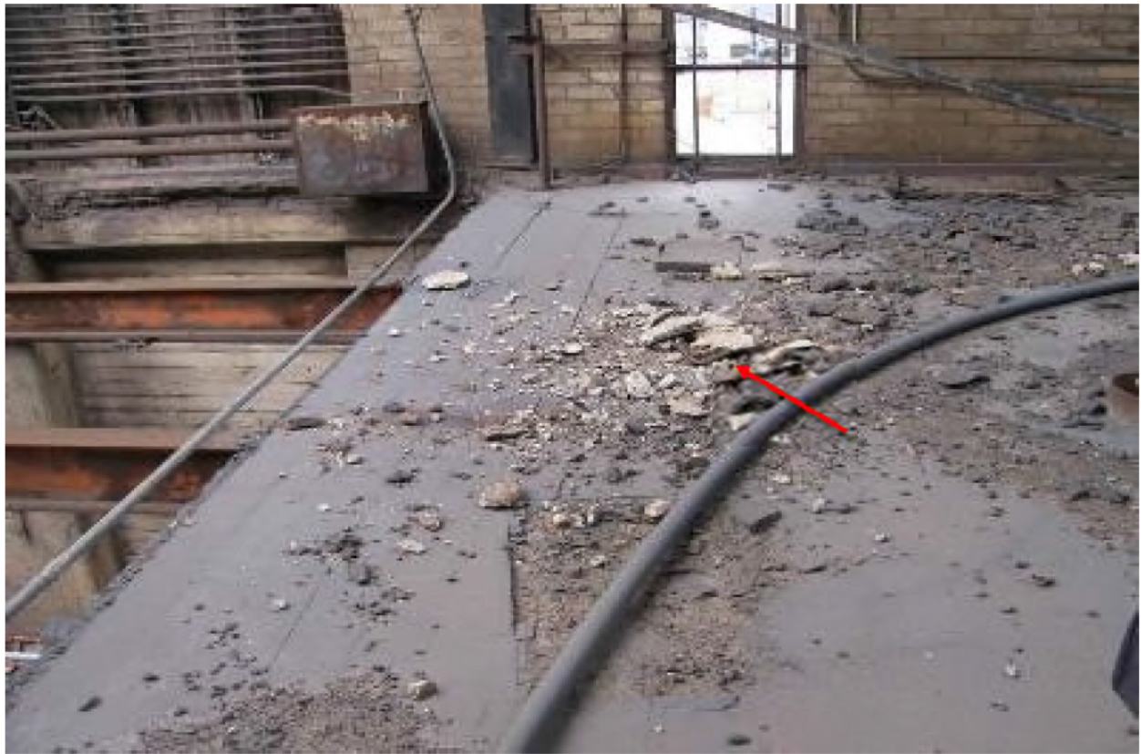
Figure 36: Unit 4 Chlorinator Building, second level “new” spalled concrete
