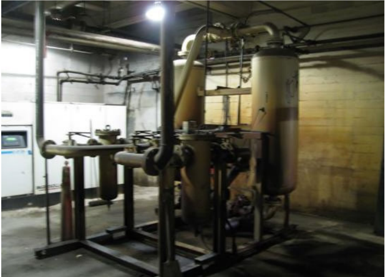
Figure 31: Unit 4 Chlorinator Building air dryer below spalling concrete
