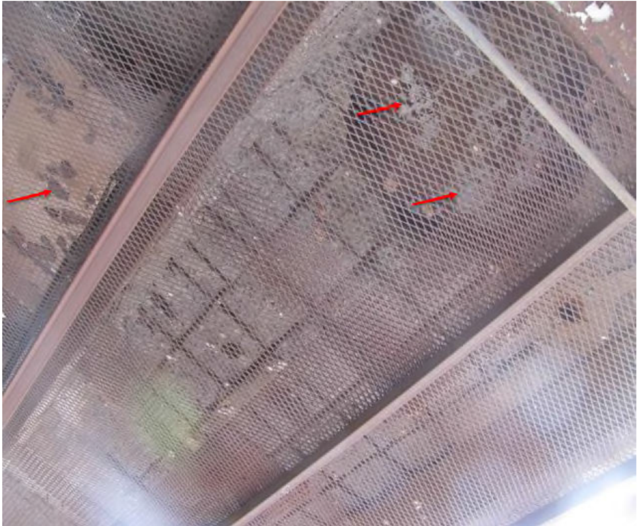
Figure 27: Unit 4 Chlorinator Building expanded metal grating retrofit under concrete actively spalling
