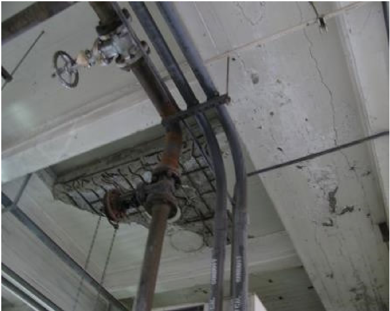
Figure 30: Unit 4 Chlorinator Building - spalling concrete above compressor
