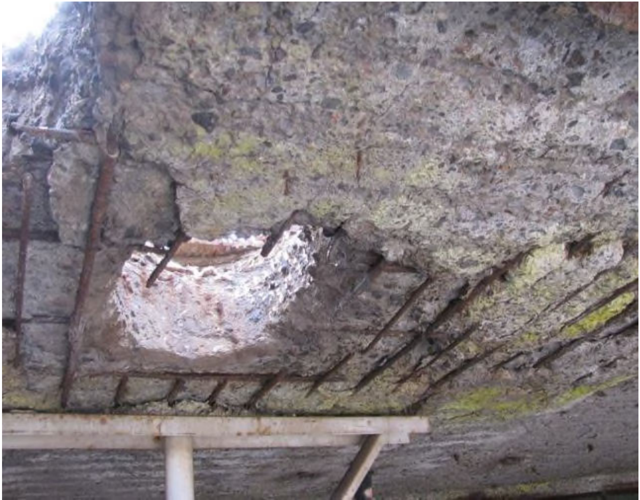
Figure 17: Curtain slab of Unit 4 Cell Floor showing typical spalling
