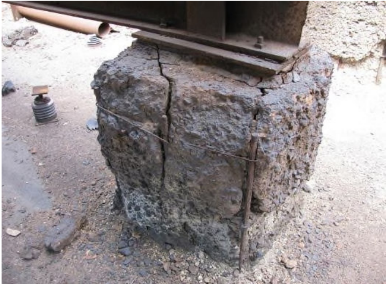
Figure 18: Unit 4 Cell Floor column pedestal, exposed rebar and severe rust and cracking
