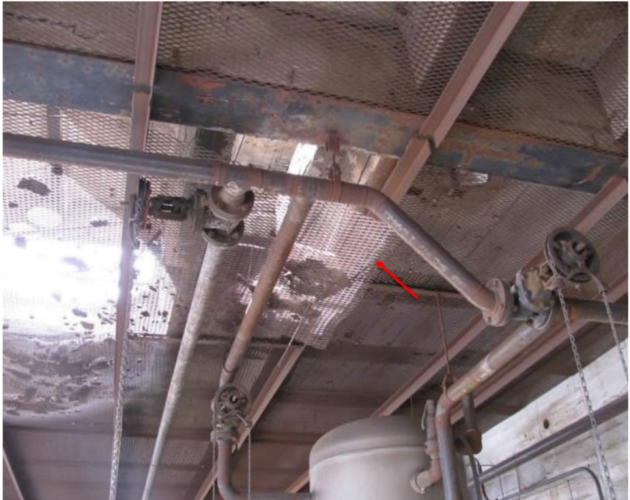
Figure 28: Unit 4 Chlorinator Building spall protection failure
