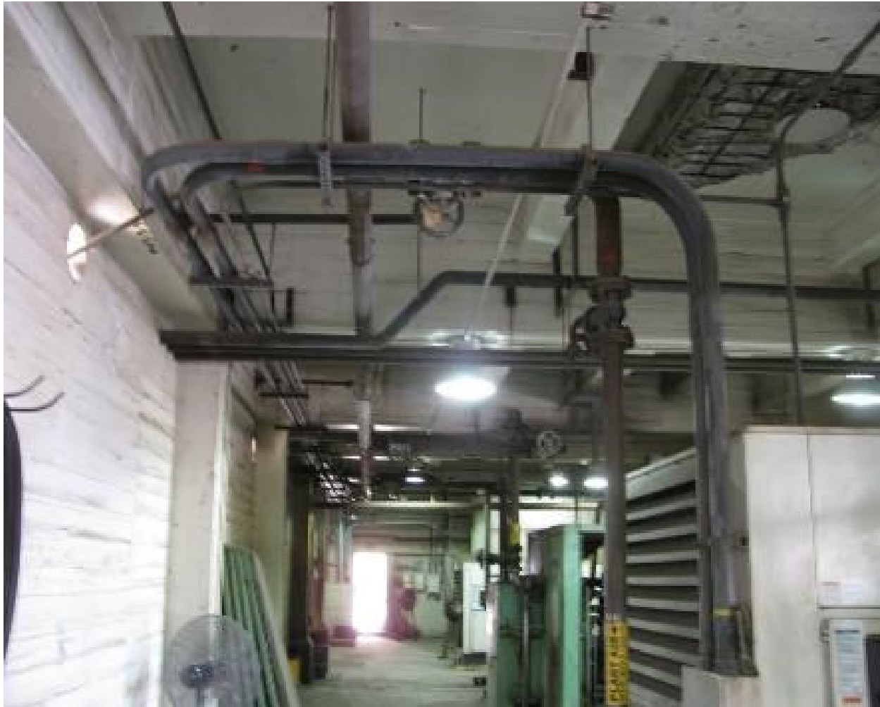
Figure 29: Unit 4 Chlorinator Building operational Compressor with active concrete spalling above
