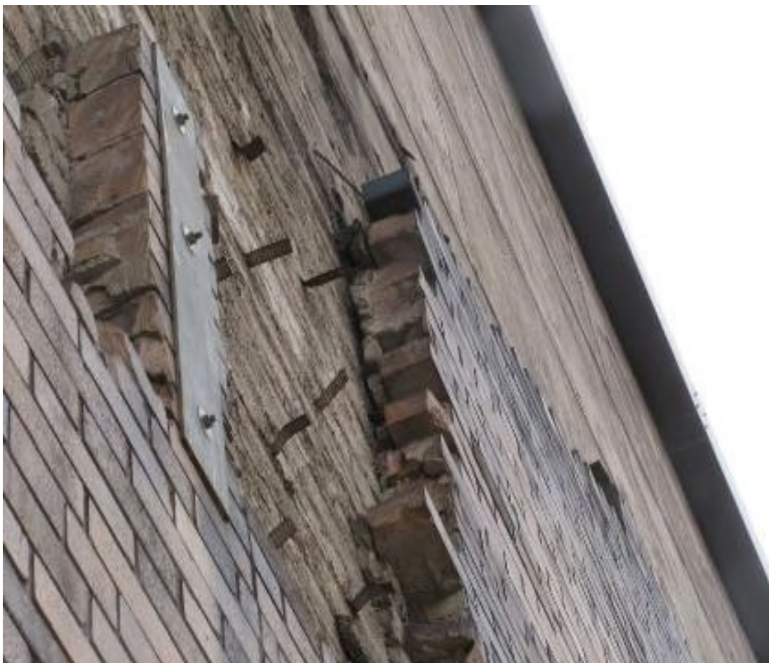
Figure 6: Loose façade bricks on the north wall of Unit 4 Substation Building
