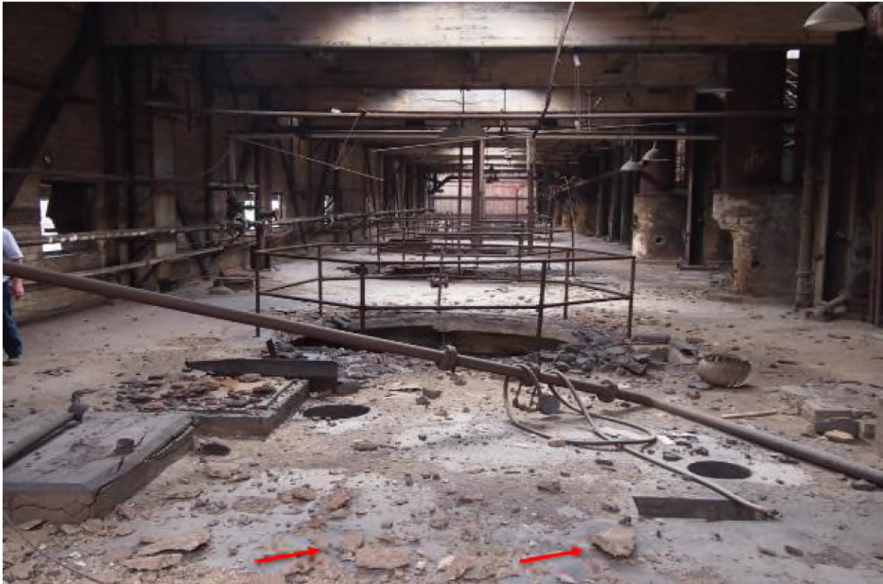
Figure 34: Unit 4 Chlorinator Building – second level
