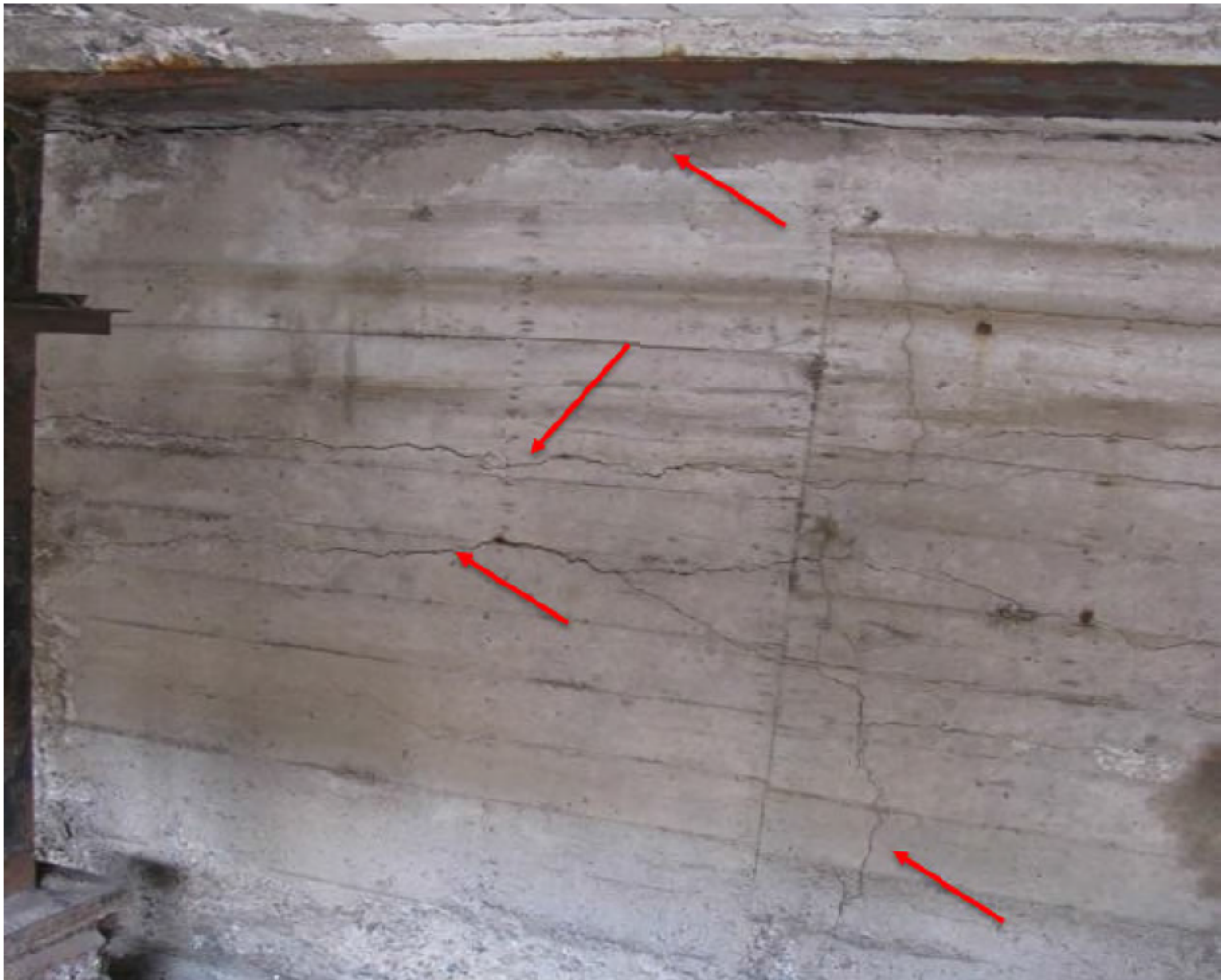
Figure 25: Horizontal cracking in the partition wall separating the Unit 4 Cell Floor Area from an air passageway
