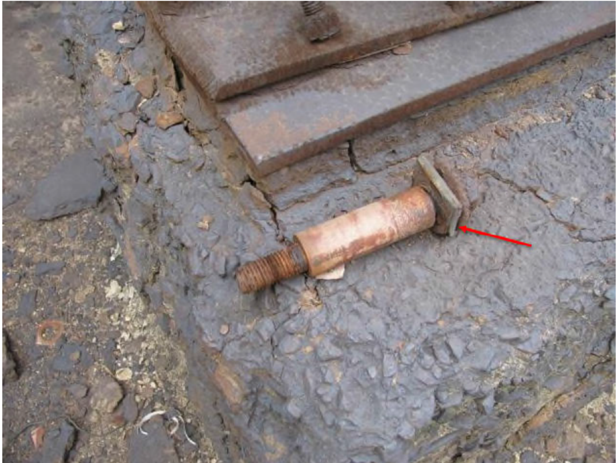
Figure 21: Anchor bolt with square washer suspected of containing asbestos
