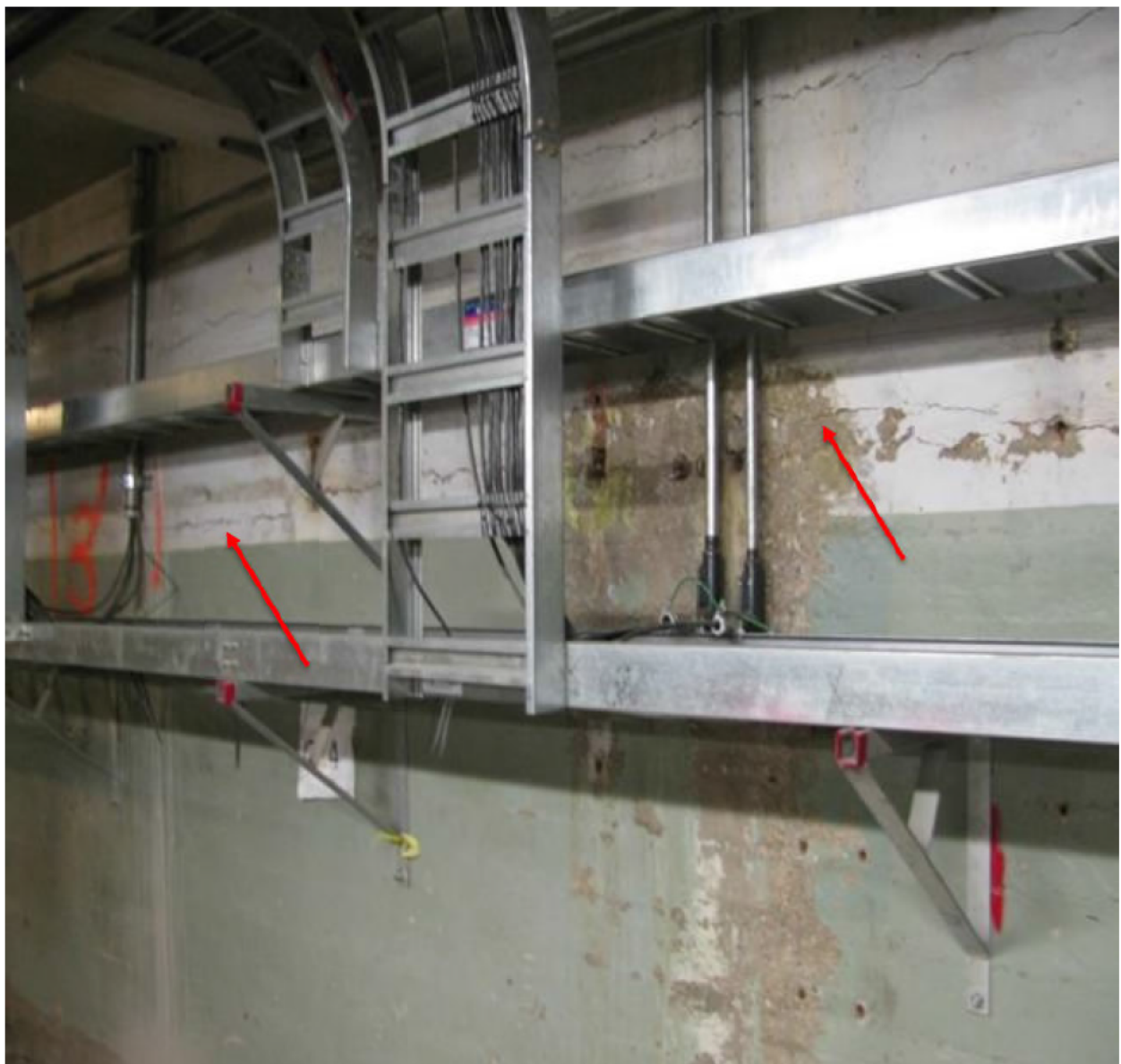
Figure 12: Horizontal cracks in basement north wall
