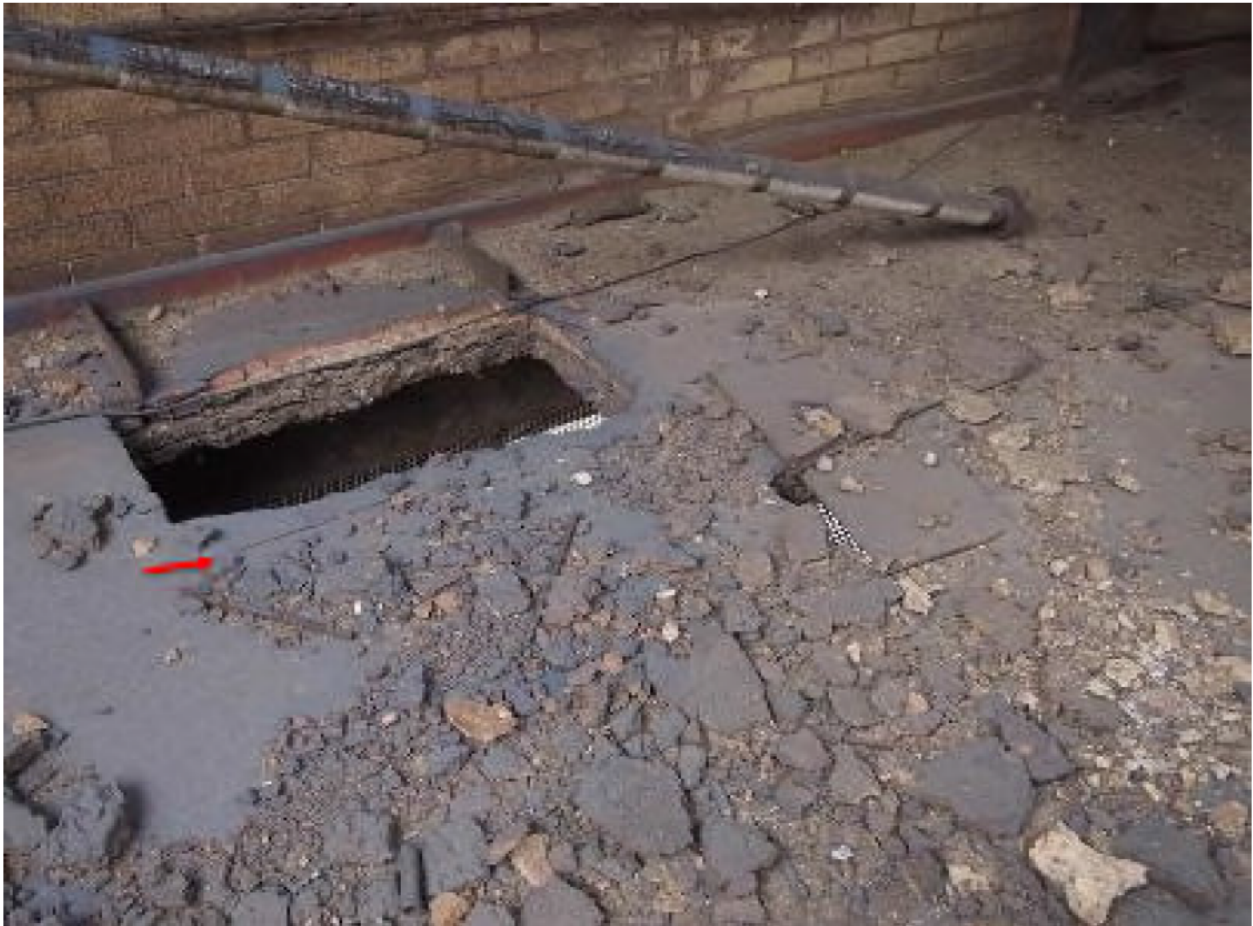
Figure 35: Unit 4 Chlorinator Building – unmarked hole in second level slab
