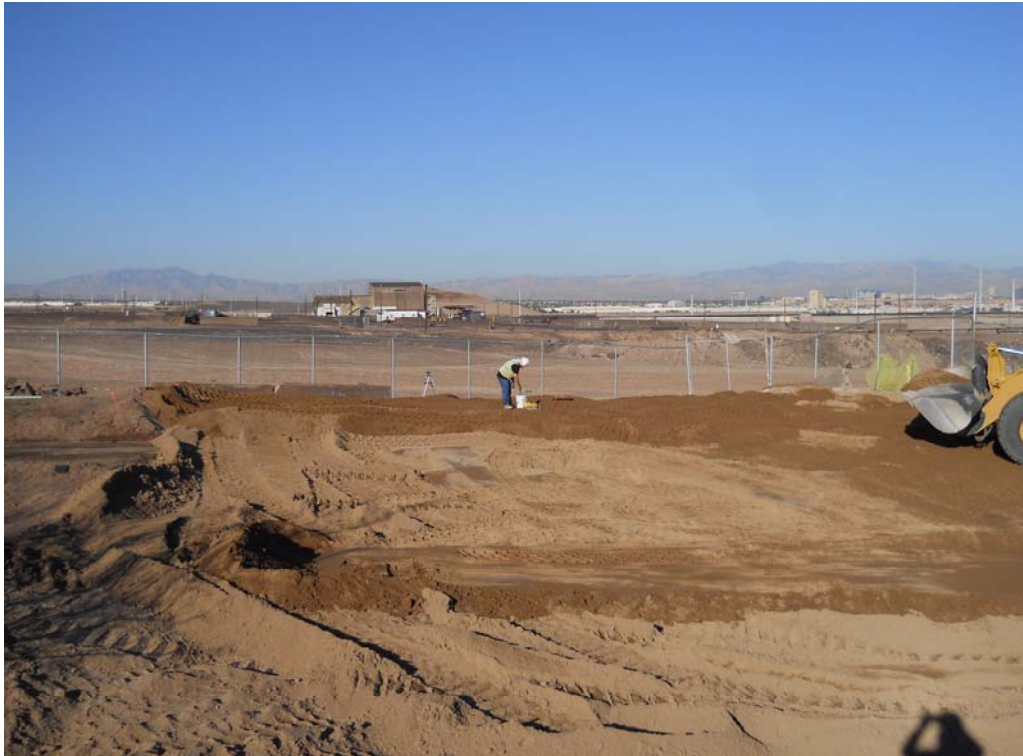
Photo 13: Facing west. Backfilling and compaction completed, final compaction testing in progress. October 14, 2013.
