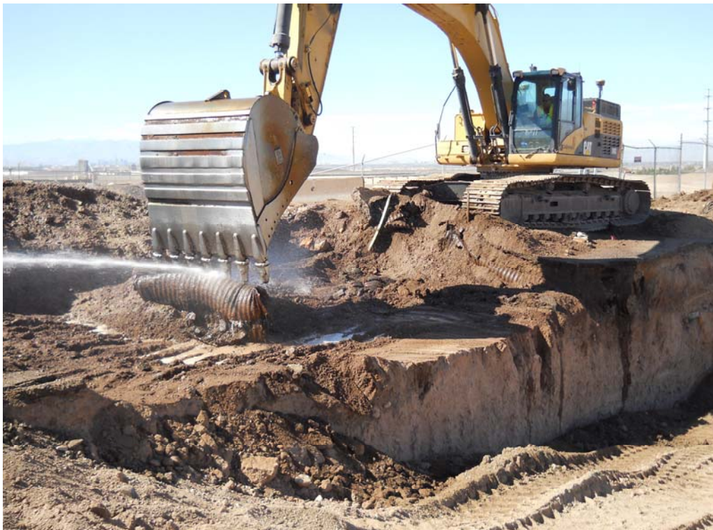
Photo 2: Facing northwest. Removal of culvert pipes from shallow soil adjacent to former structures. October 1, 2013.
