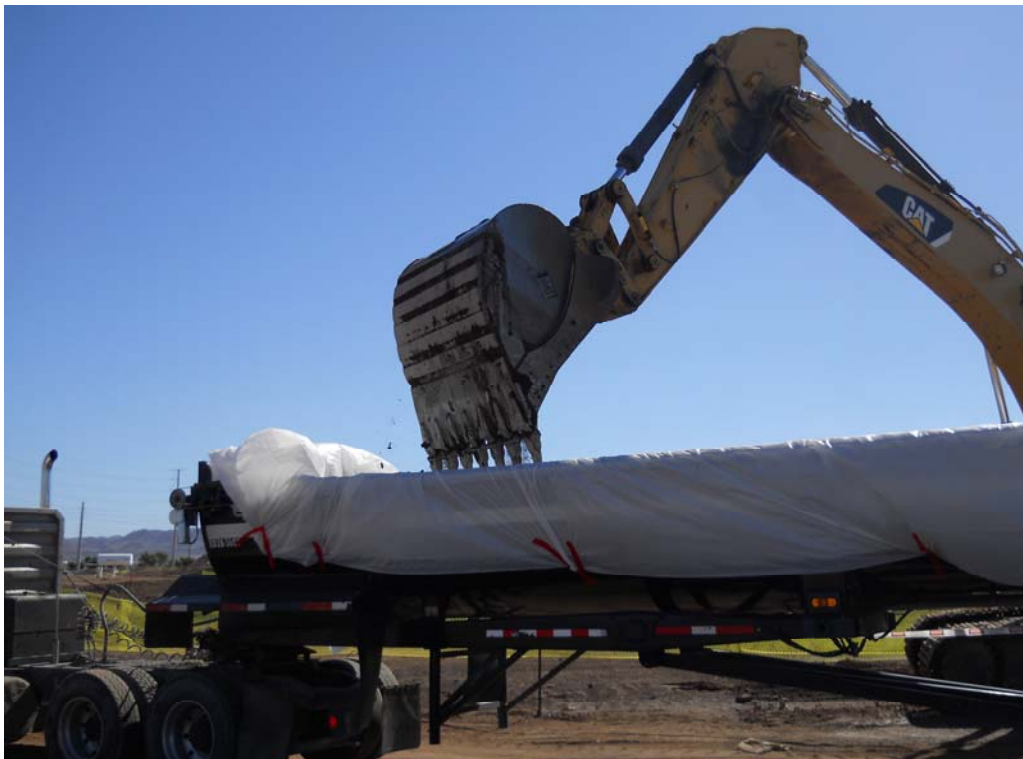
Photo 4: Loading of asbestos-impacted soil into end-dump trailer lined with plastic sheeting. October 2, 2013.
