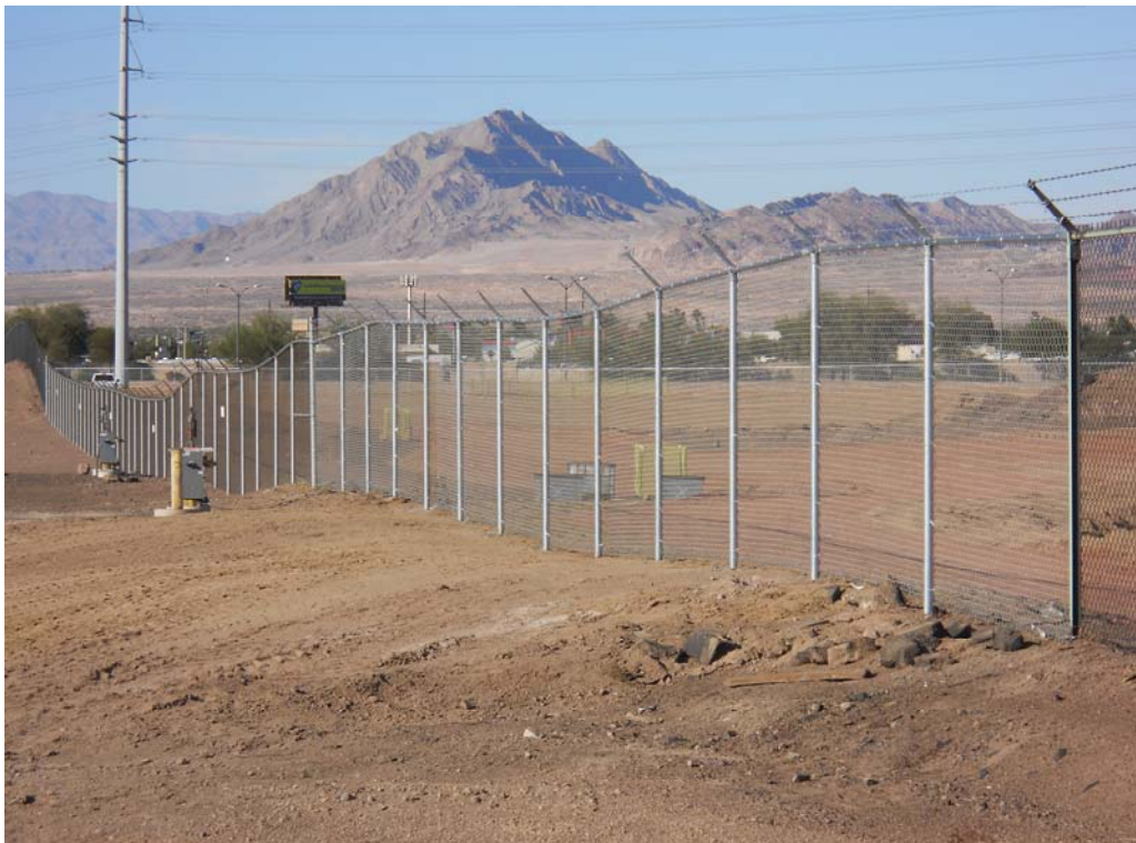
Photo 18: Facing northeast. New perimeter security fencing has been installed to complete the project. October 21, 2013.
