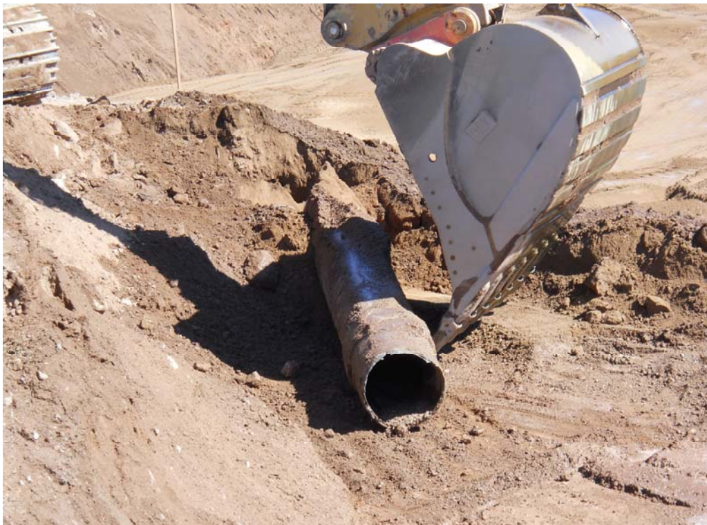
Photo 8: Removal of last remaining portion of Pittman Bypass Pipeline within excavation area. October 4, 2013.
