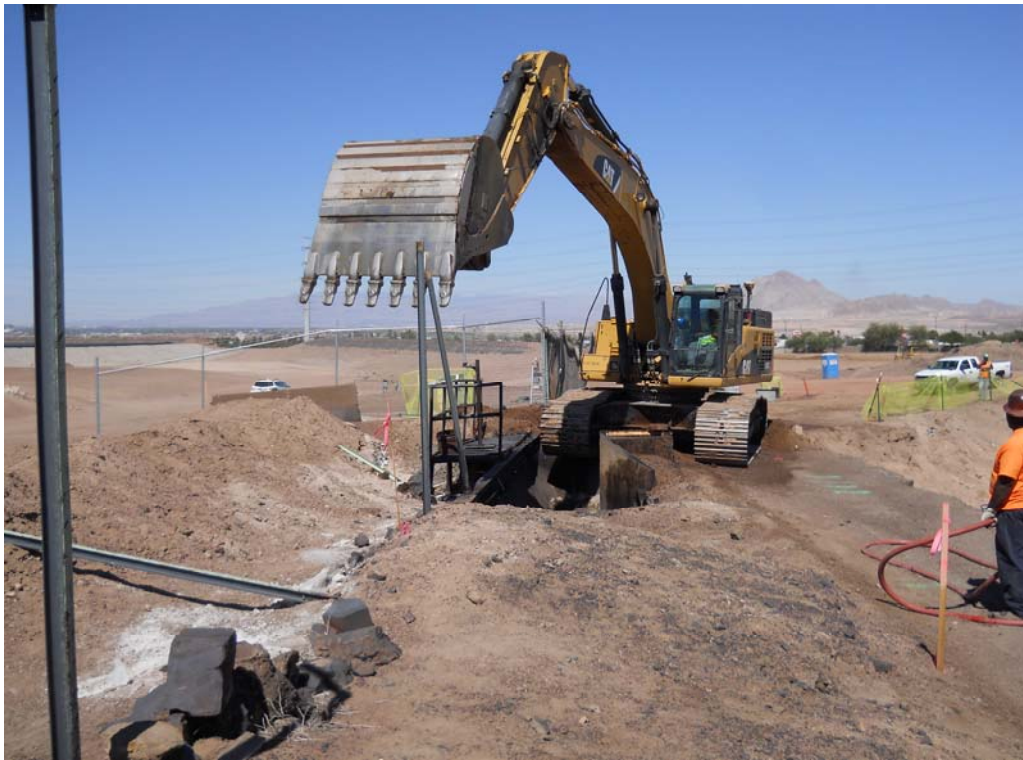
Photo 1: Facing north. Removal of structures at east end of former Beta Ditch. October 1, 2013.
