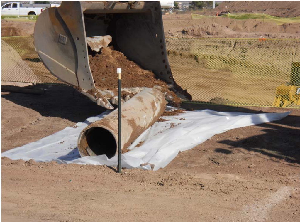
Photo 5: Facing northeast. Containing transite pipe (containing asbestos) within plastic sheeting for disposal. October 3, 2013.
