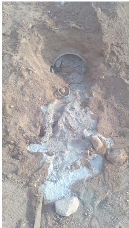
Photo 10: End of Pittman Bypass Pipeline terminating at excavation boundary. Pipeline was sealed with concrete and mortar. October 7, 2013.
