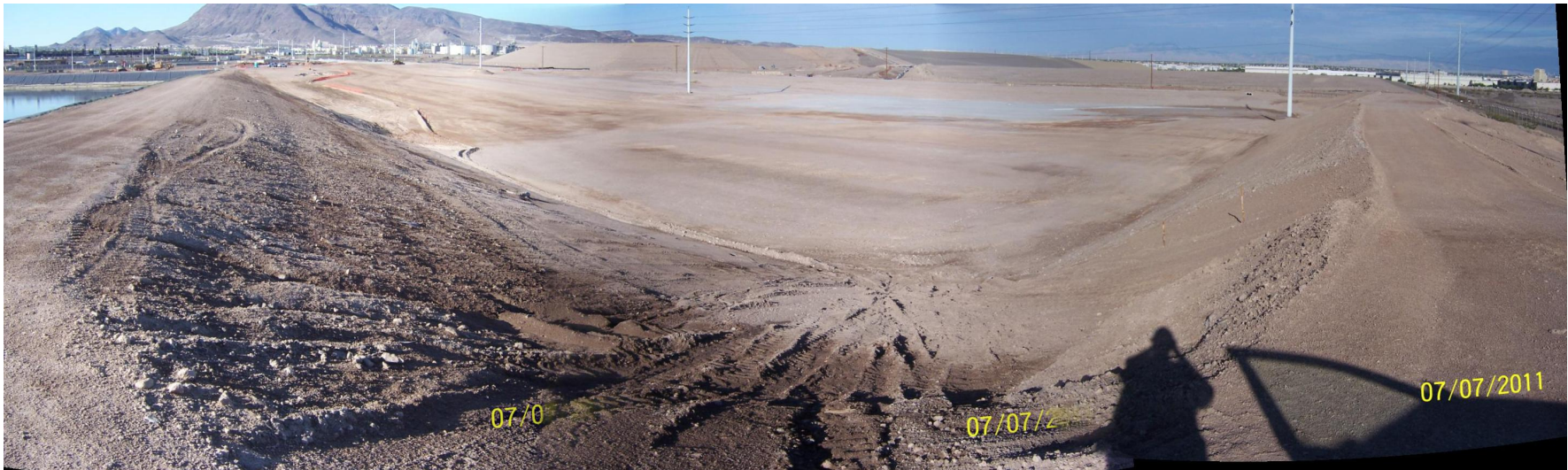
West RZ-D-1 to 7 Restoration Grading after Polygon Backfill Ready for Placement of Slope Treatment
