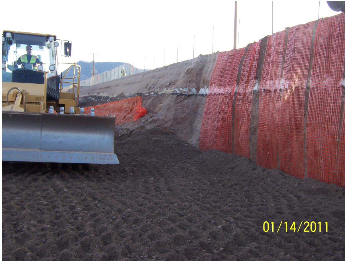
West RZ-D-1 to 7 Special Excavation of the West Property Line to Vertical And then Placement of Orange Fencing before Placing Backfill
