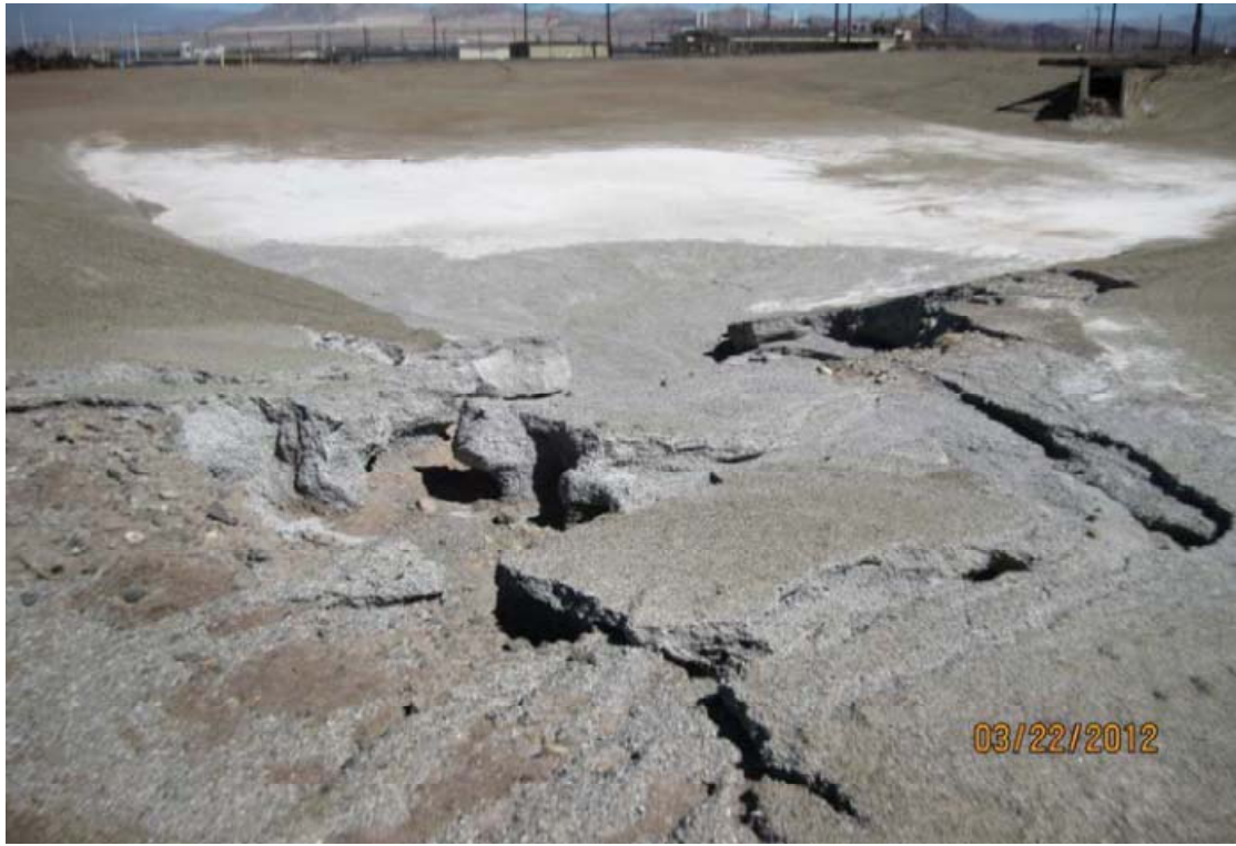
Photo 3: Large washout area looking northeast.
