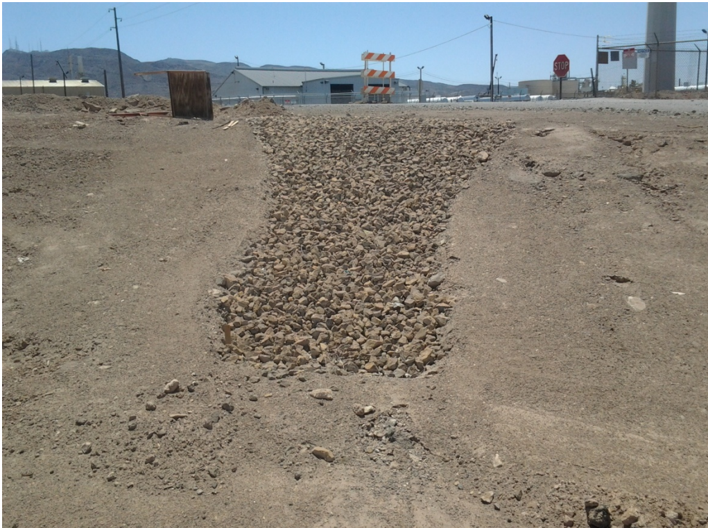
Photo 1: Typical Energy Dissipating Channel – Geotextile Fabric Covered with approximately 8” of Stone
