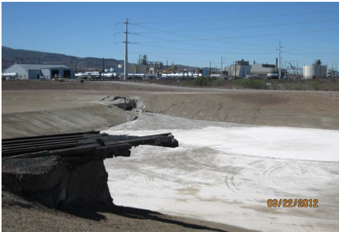
Photo 4: Looking southwest over rail crossing at large wash out.
