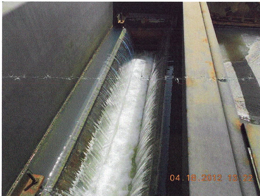
Fig. 9 – DAF Effluent (to filter)
