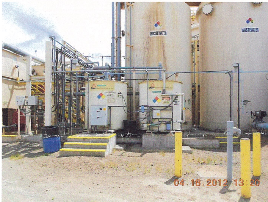
Fig. 7 – GAC Odor Control for Gaseous Emissions
