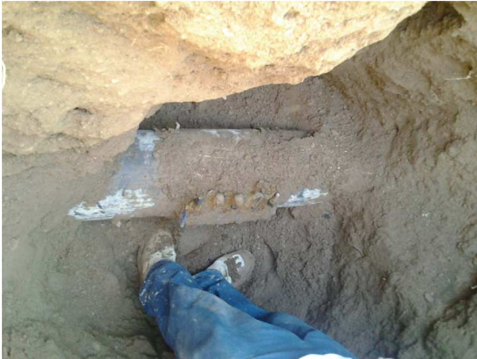
Failed collar on effluent pipe 2/24/12 10:30 AM
