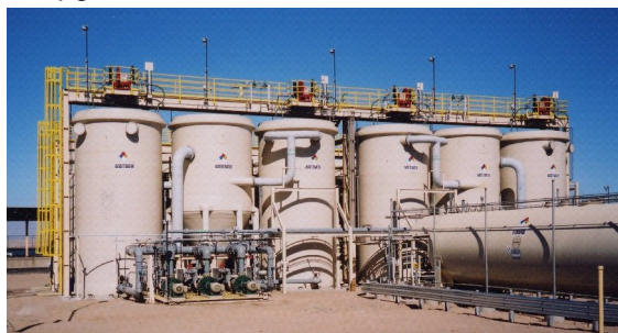
Biological Treatment Plant for Groundwater
