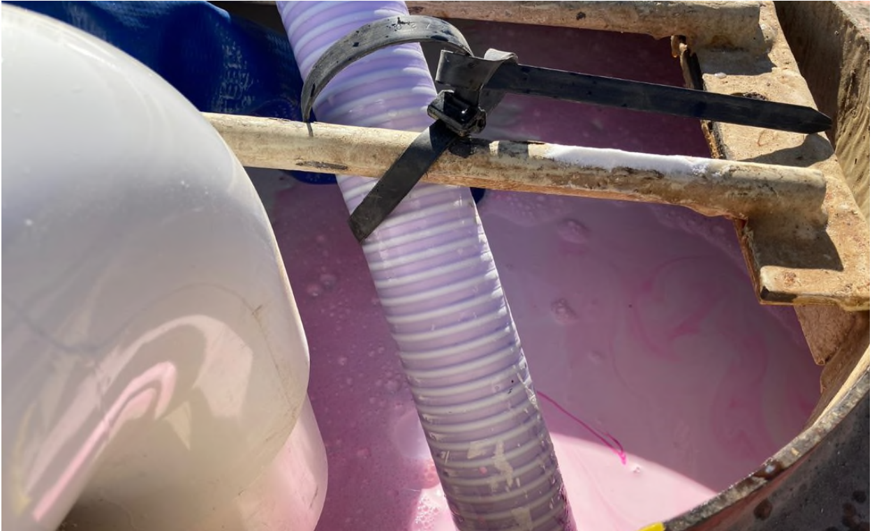
Adding and mixing rhodamine into batch mixing tank for Injections into alluvium
