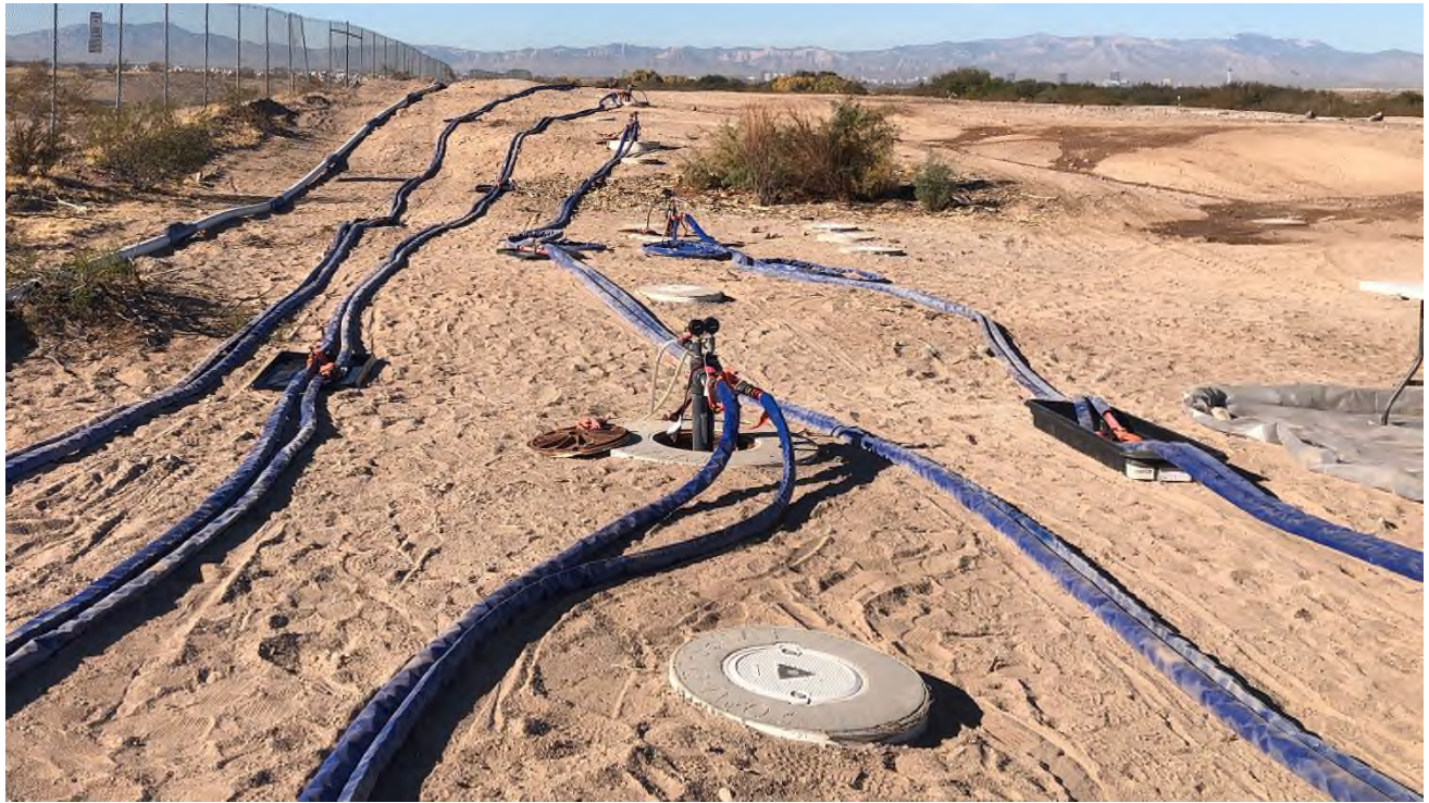
Injection well lines connected from the injection manifolds to the individual injection wells.
