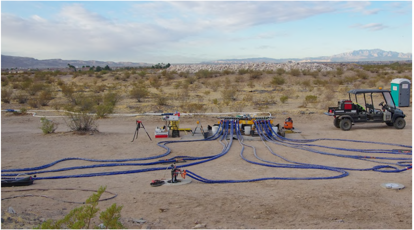
Fully connected injection well transect line within Zone 1 - UMCf.
