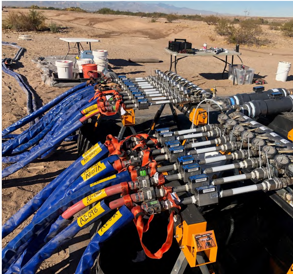
Manifold Flow Meters/Totalizers and Pressure Gauges; Lines Labeled with Injection Well Name
