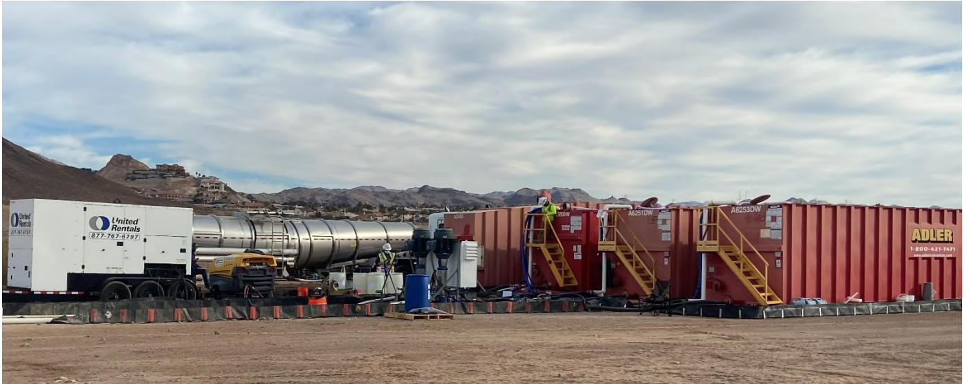
Deliveries of EOS PRO product are off-loaded into a 21,000-gallon frac tank (left). Three 16,400-gallon frac tanks are used for batch mixing of the injectate solution (right).
