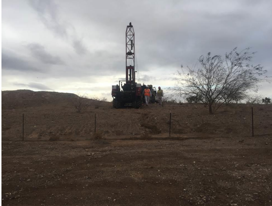
Photo 1. Borehole B-8, View looking west in location of the Historic Lateral Pump Station.
