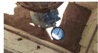
Pressure gauge at Station 174+20
