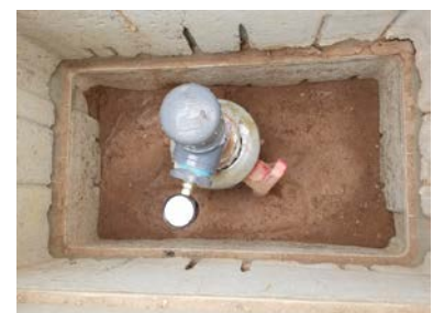
Pressure gauge at Station 185+60
