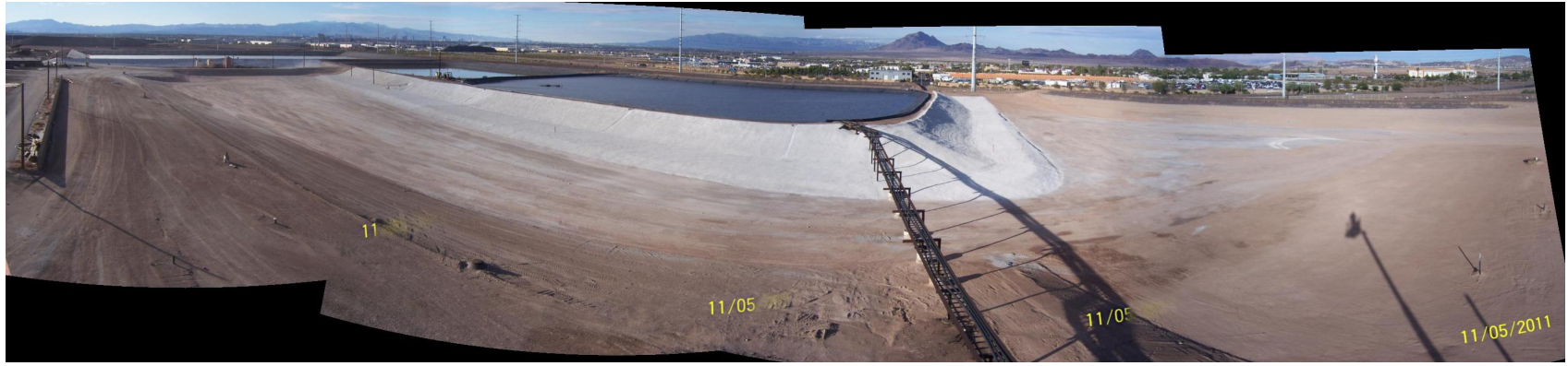
East RZ-D-15 to 24A Finished Grade of Basin with Slope Treatment Placed
