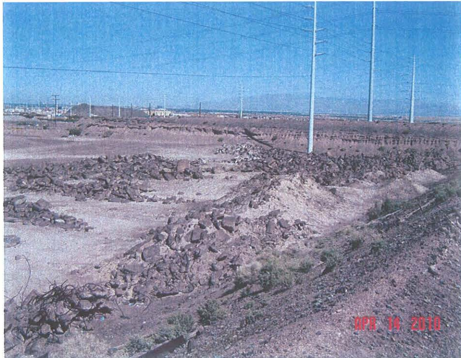
Photo 17 – West side debris pile looking northwest from top of hill.
