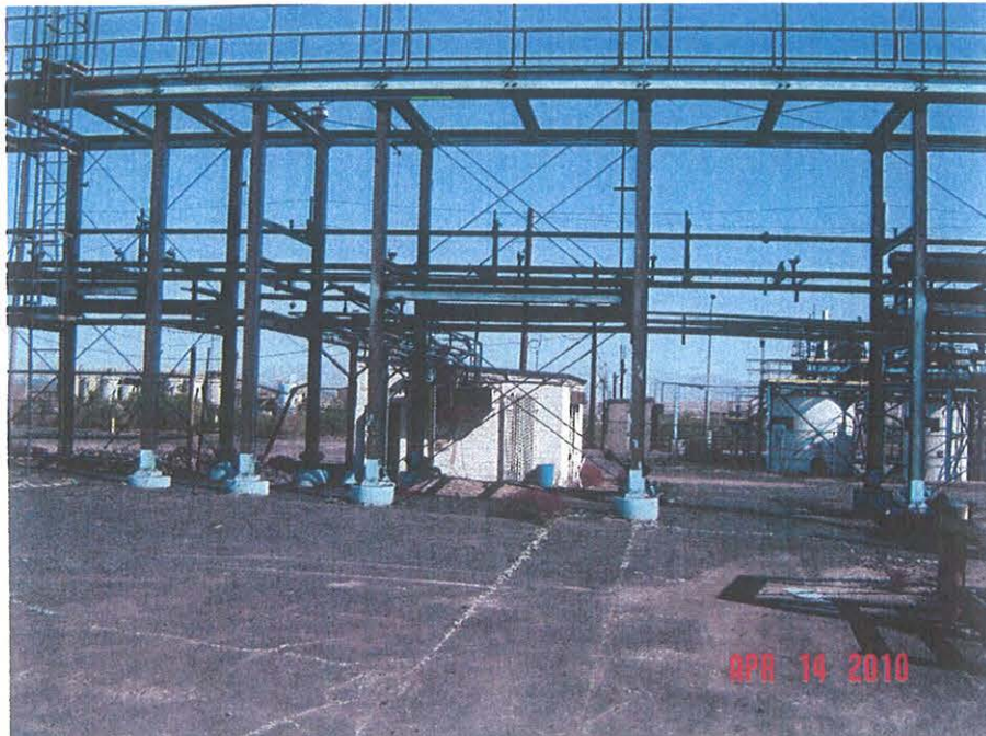
Photo 4 – Small building in center of picture has panels that are non-asbestos on north side of building
