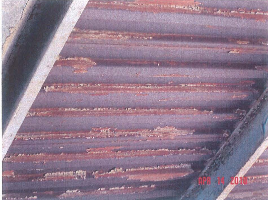
Photo 5 – Loose and flaking lead containing paint on the underside of the roof deck.
