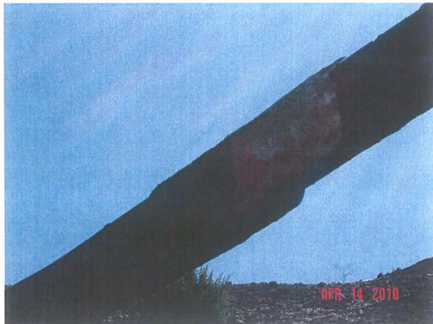
Photo 10 – West side debris pile. Close-up of asbestos pipe wrap.
