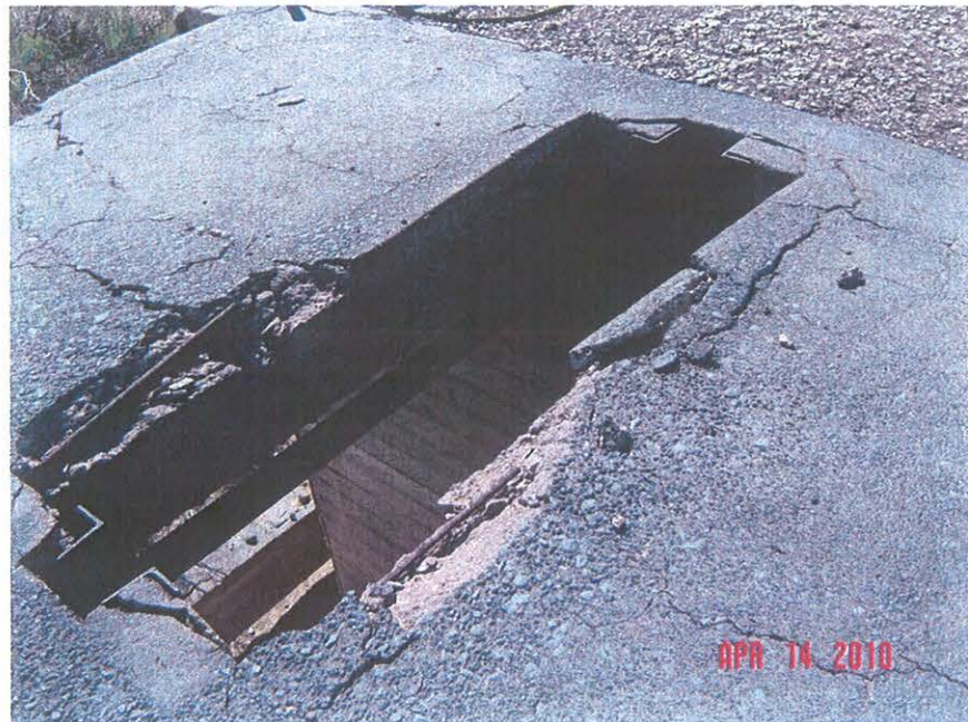
Photo 20 – West side debris pipe. Pipe under concrete at far south of hill.
