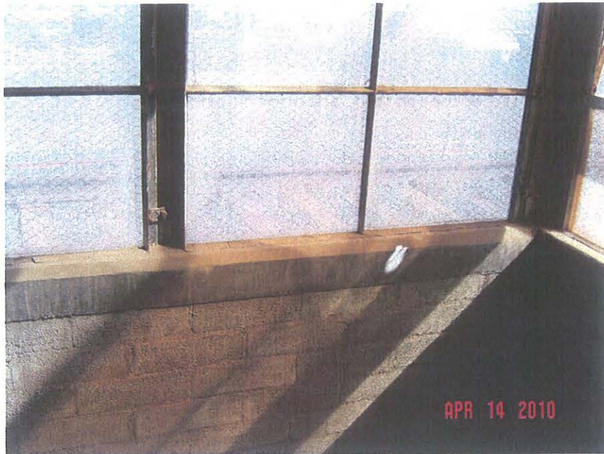
Photo 3 – Interior of windows seen in above building contains asbestos window putty.
