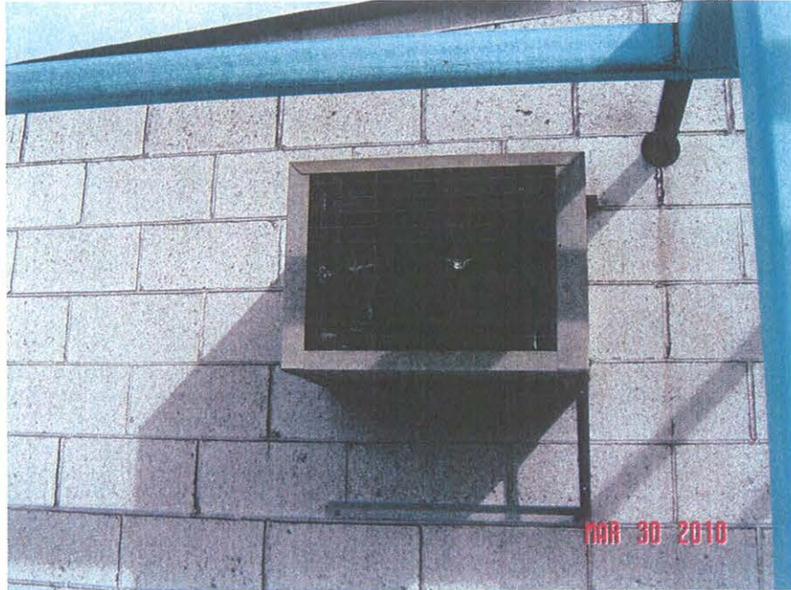
Photo 3 – AC unit on calciner building.
