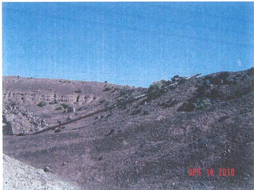
Photo 14 – West debris pile with pipe on side of hill. Pipe contains asbestos pipe wrap.
