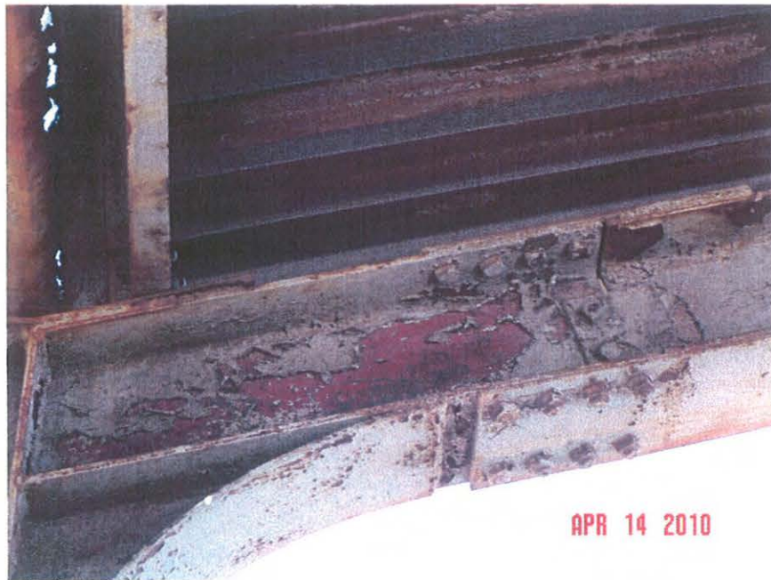
Photo 6 – Loose and flaking lead containing paint on beam of railroad depot.
