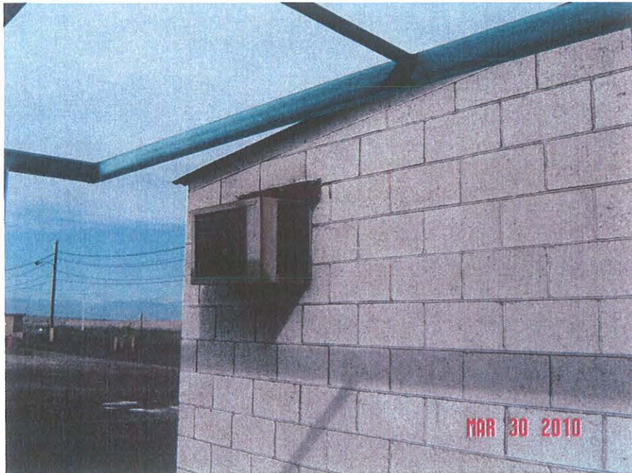
Photo 4 – AC unit on calciner building
