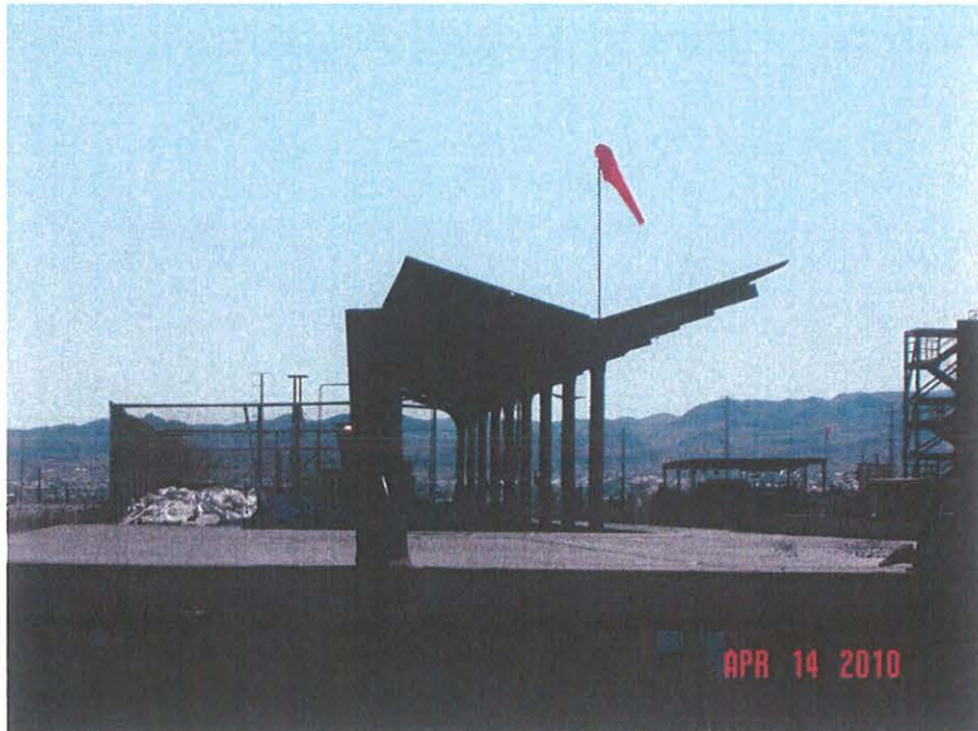
Photo 4 – Rail road depot has loose and flaking lead containing paint.
