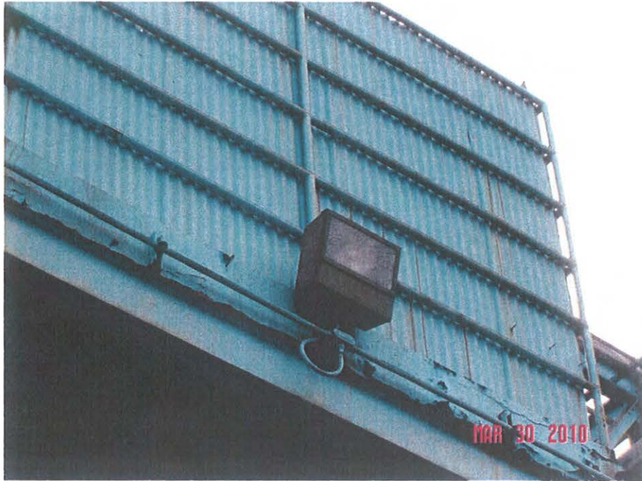
Photo 7 – Mercury containing light, close up view
