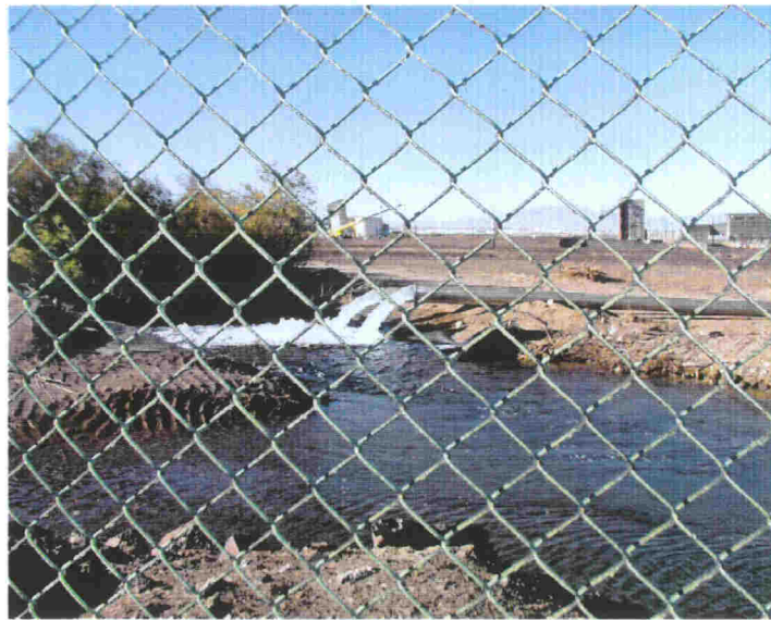
Photo 1. Discharge pipe flow into the Beta Ditch
