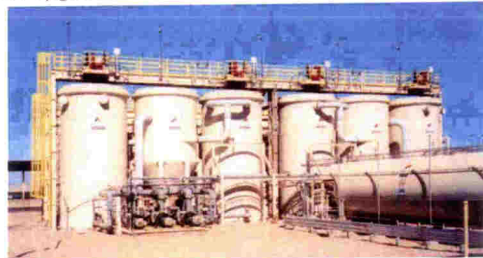
Biological Treatment Plant for Groundwater
