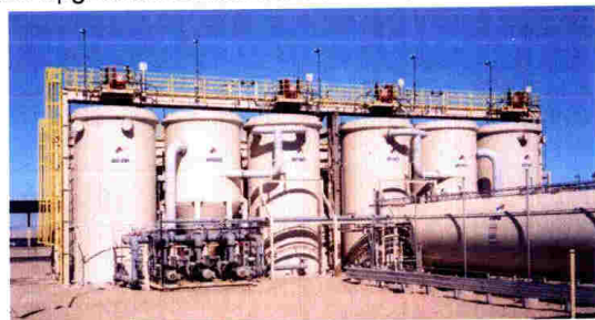
Biological Treatment Plant for Groundwater
