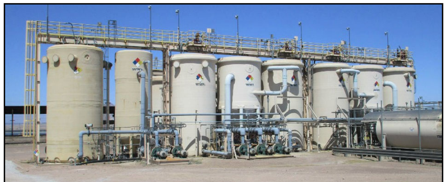
Groundwater Treatment System at the NERT Site
